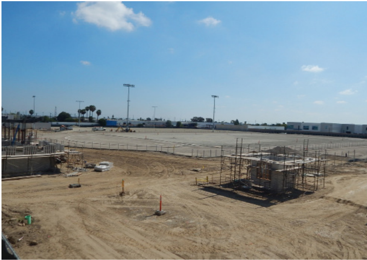
Photo by Stephanie Martinez Construction on the new Stadium, as of October 2018.
