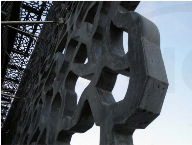
Fig. 6.9—MuCEM general overview and close-up of facade panels (photos courtesy of Ben Graybeal).
