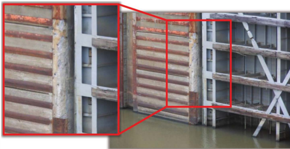
Fig. 6.10a—Typical damage vertical armor plate component at miter gate recess in inland navigation lock structure (photo courtesy of Robert Moser).
