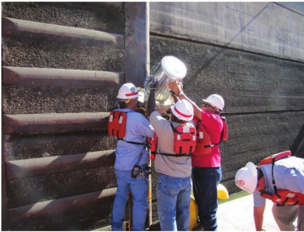
(a) Placement of repair material by pouring through ports (photo courtesy of Robert Moster)
