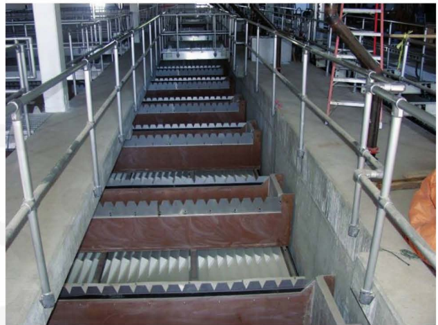
Fig. 6.11a—UHPC troughs for the Gold Bar Wastewater Treatment Plant, Edmonton, AB, Canada (McCraven 2007).
