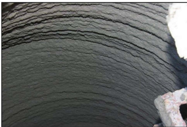
Fig. 6.11b—Rotating spray nozzle and finished sprayed surface (photos courtesy of City of Naperville).
