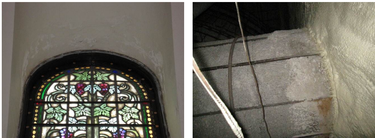
Figure 12. Moisture issues at chapel windows (Brennan 2011)
