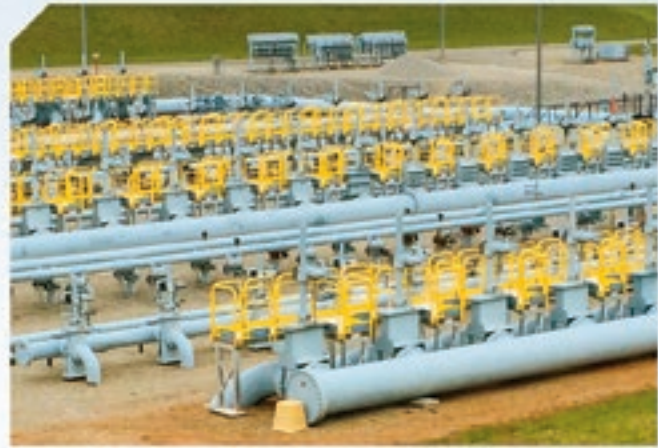
Safely and efficiently access multiple valves.
