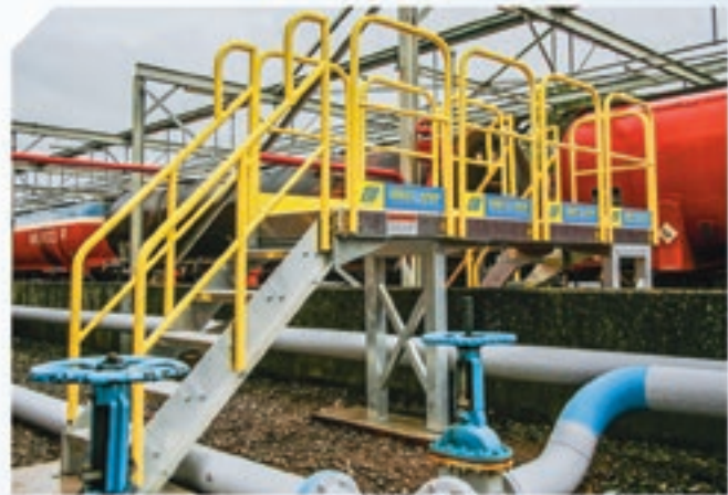
Access over and across multiple obstructions safely.
