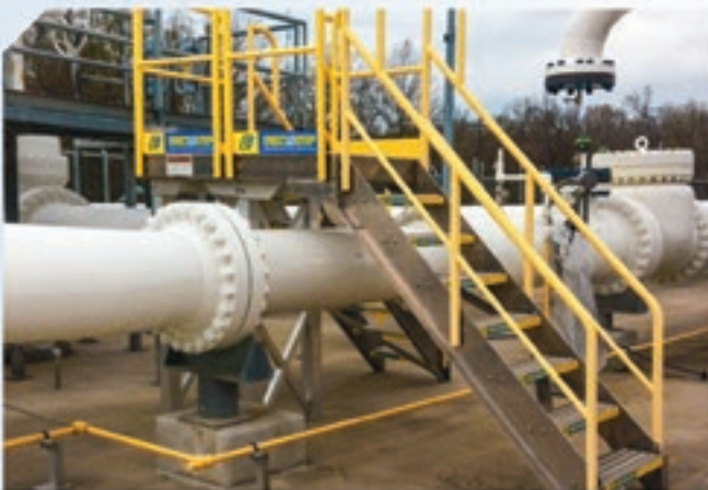
Large oil pipeline cross over.
