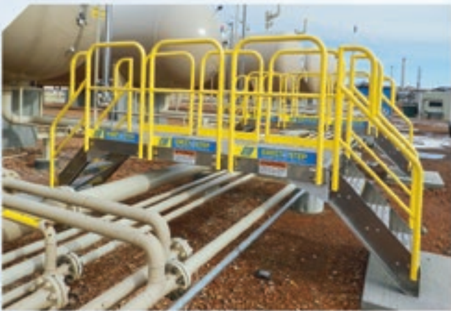
Propane gas lines no longer a safety issue.
