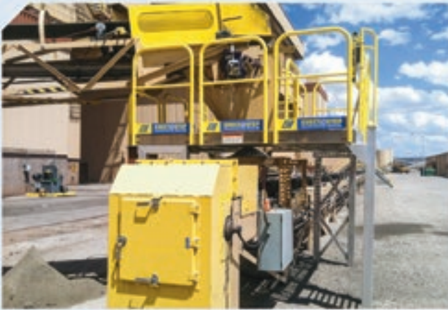
Work safely on all four sides of this conveyor motor at this power generation station.
