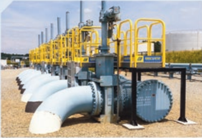
Safe valve access.
