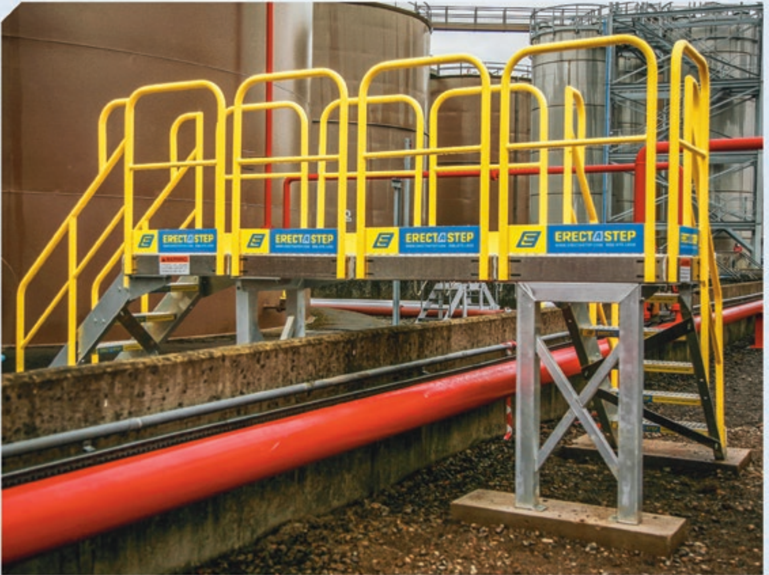
Safely access storage tanks in all weather conditions.
