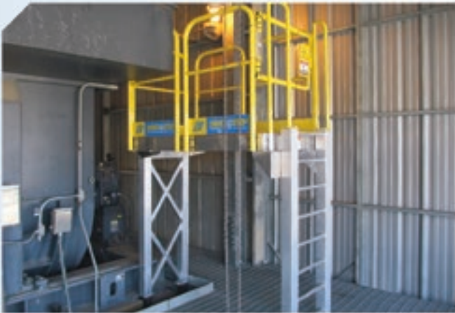
Changing these industrial filters has never been safer.
