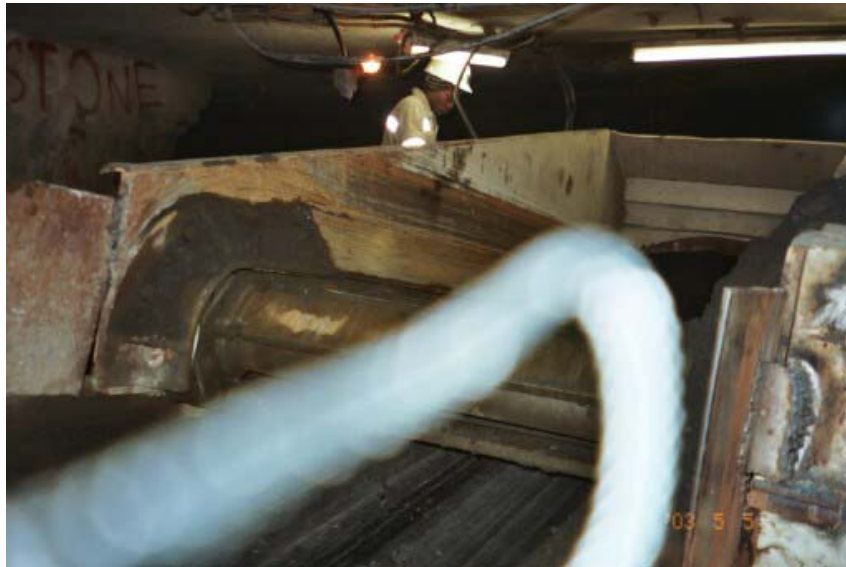
Conveyer belt for ore transportation
