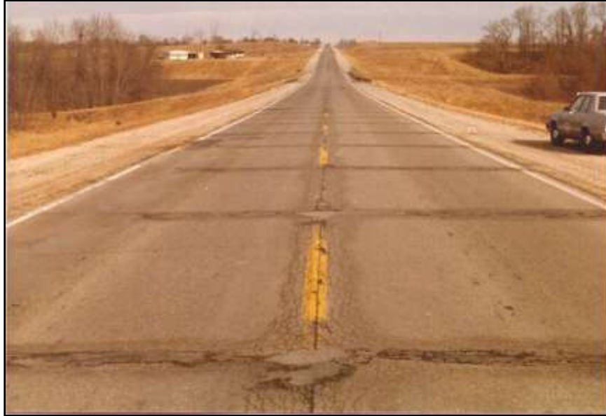
Figure 9 - D-Cracking on U.S. 218 MP 46 - 1970s
