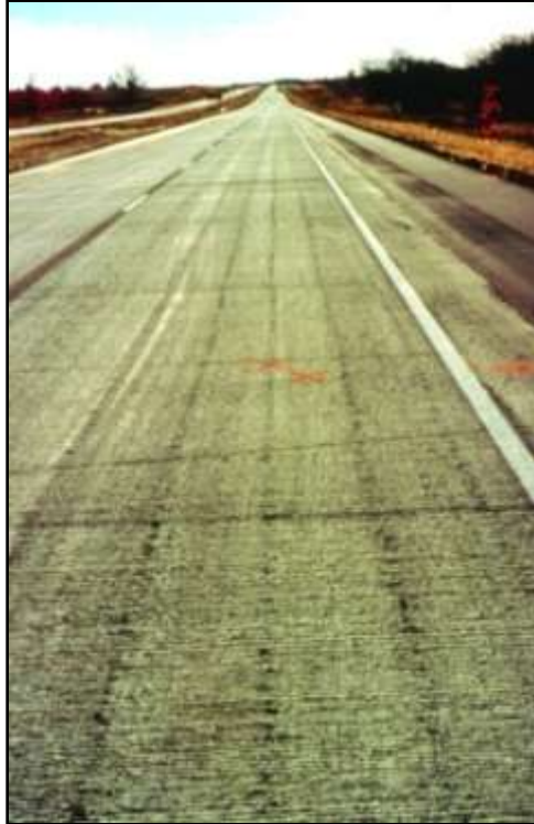
Figure 38 - Vibrator trails in pavement - Dallas County
