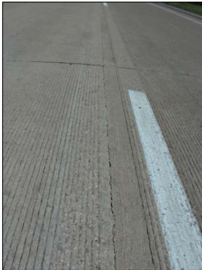
Figure 62 - Hairline crack on knifed joint
