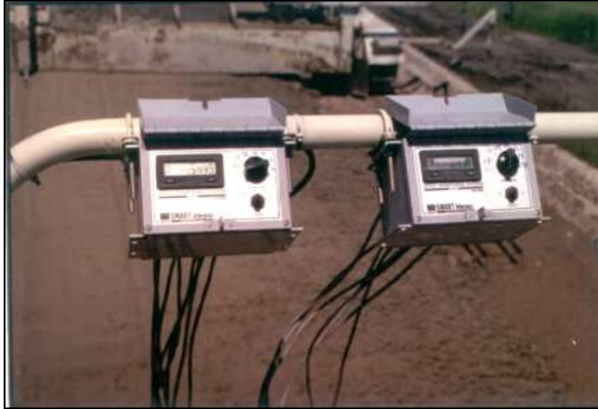
Figure 39 - Vibration monitoring equipment
