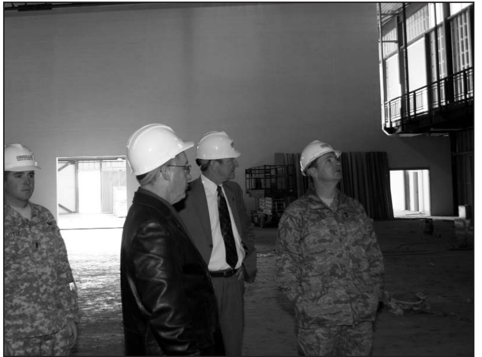
Maj. Gen. Tod Bunting, the adjutant general; Dr. Tom Bryant (second from the right), president of Pittsburg State University, John D. Patterson, vice president, Pittsburg State University; and 1st Lt. Michael Liotta (left) tour the new armory being built on the grounds of Pittsburg State University. The groundbreaking ceremony for the building was held in May and it is expected to be finished in the spring of 2008. This is the first National Guard armory in Kansas that has ever been located on a university campus. The Kansas National Guard will utilize 39,000 square feet of the 97,000 square foot facility for offices, locker rooms, kitchen and training and support areas, plus an exterior compound and maintenance bay. The university's portion will be used for offices for the Departments of Health, Physical Education and Recreation and Military Science/Reserve Officer Training Corps (ROTC) along with the PSU Student Recreation Center. The recreation center will include cardio equipment, free weights, an aerobics room and gymnasiums. Joint use areas will include an assembly hall, fitness center and classroom spaces. (Photo by Jane Welch)
