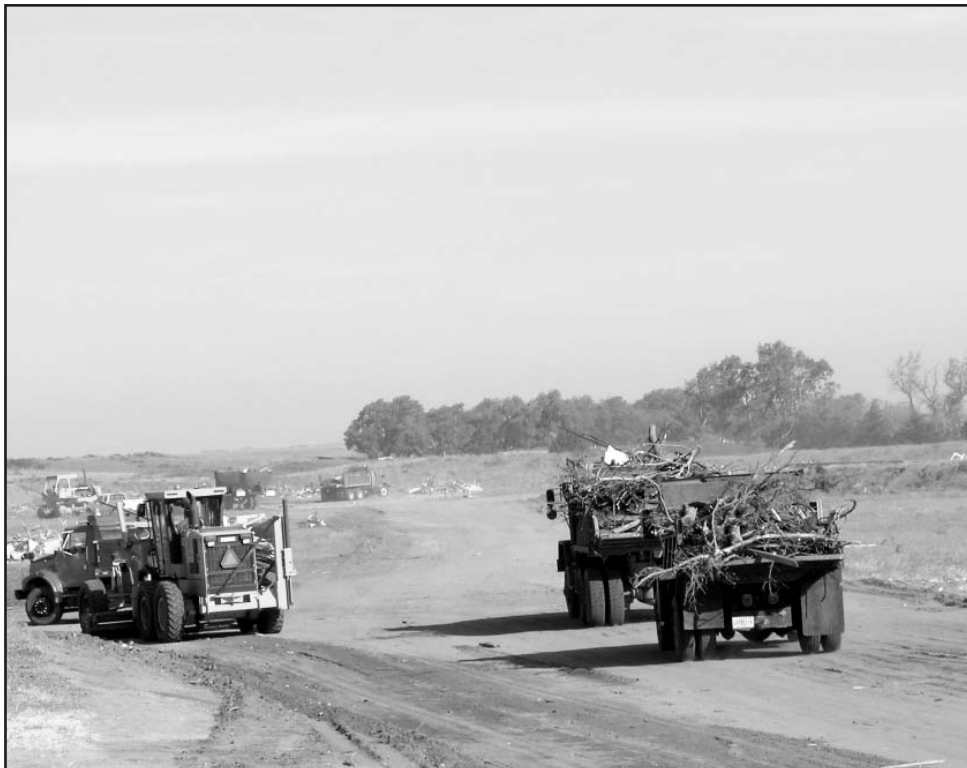
Two more loads of debris head toward the landfill from Greensburg. (Photo by the 102nd Military History Detachment)
