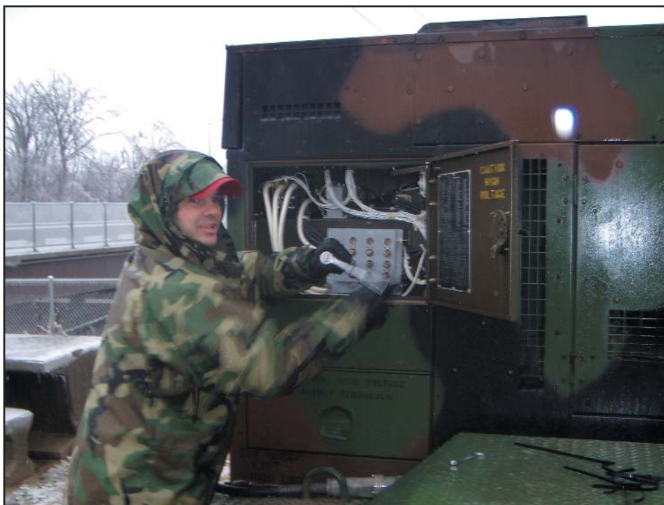
Tech. Sgt. Michael Balevre, 134th Air Control Squadron, makes adjustments on a generator supplied to an ice-stricken community during the December ice storms that swept the state. (Photo provided)
