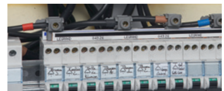
^ Distribution via supply busbars
