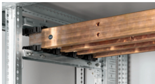
^ Main busbar at the top of the enclosure with 2 copper bars per pole
