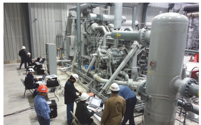
Figure 9: First PAN Manifold unit undergoing extensive thermodynamic performance testing.
