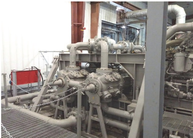
Figure 12: Second PAN Manifold unit installed (with work platforms) – right side view.
