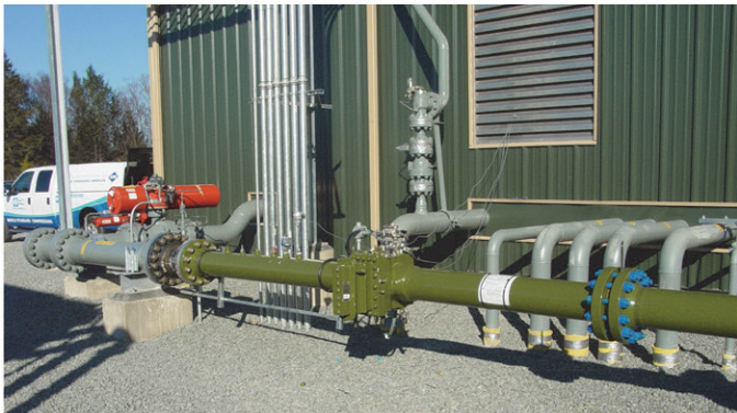
Figure 10: AGA flow meter in suction line to PAN Manifold unit, used for performance testing.
