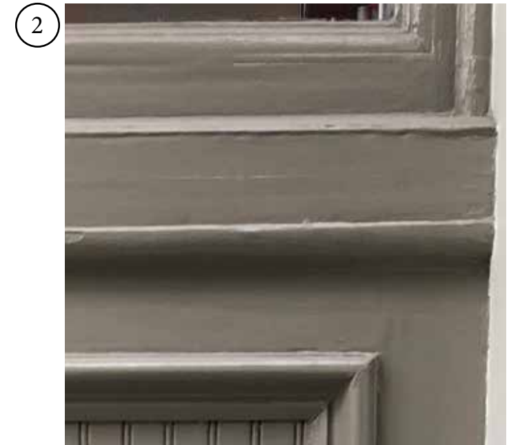
EXISTING HORIZONTAL PAINTED TRIM DOES NOT MATCH OTHER STOREFRONT WINDOW BAYS WITH CAST IRON TRIM
