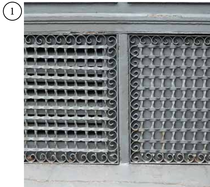
EXISTING PAINTED BULKHEAD LOUVER/METAL GRILL WITH PLYWOOD OR DIAMOND PLATE BACKER TO REMAIN
