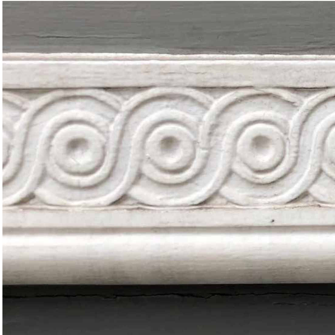
PHOTO OF EXISITING HORIZONTAL CAST IRON TRIM
