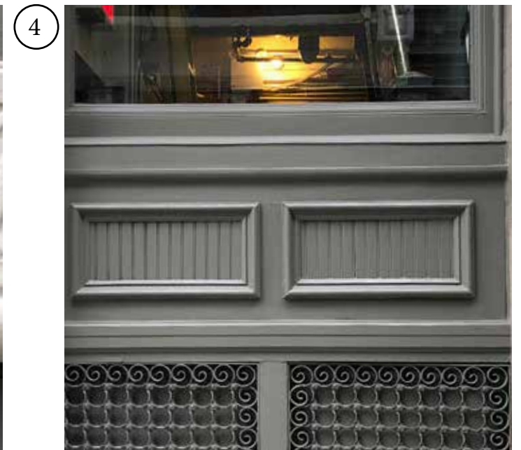
EXISTING BAY AT 84 WOOSTER - MISSING DECORATIVE CAST IRON SILL. TO BE REPLICATED IN LIKE KIND OUT OF WOOD
