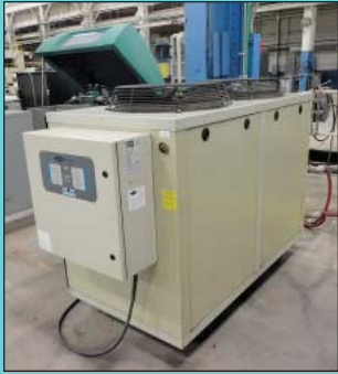
Thermal Care Model SQ2A0804 Portable Chiller
