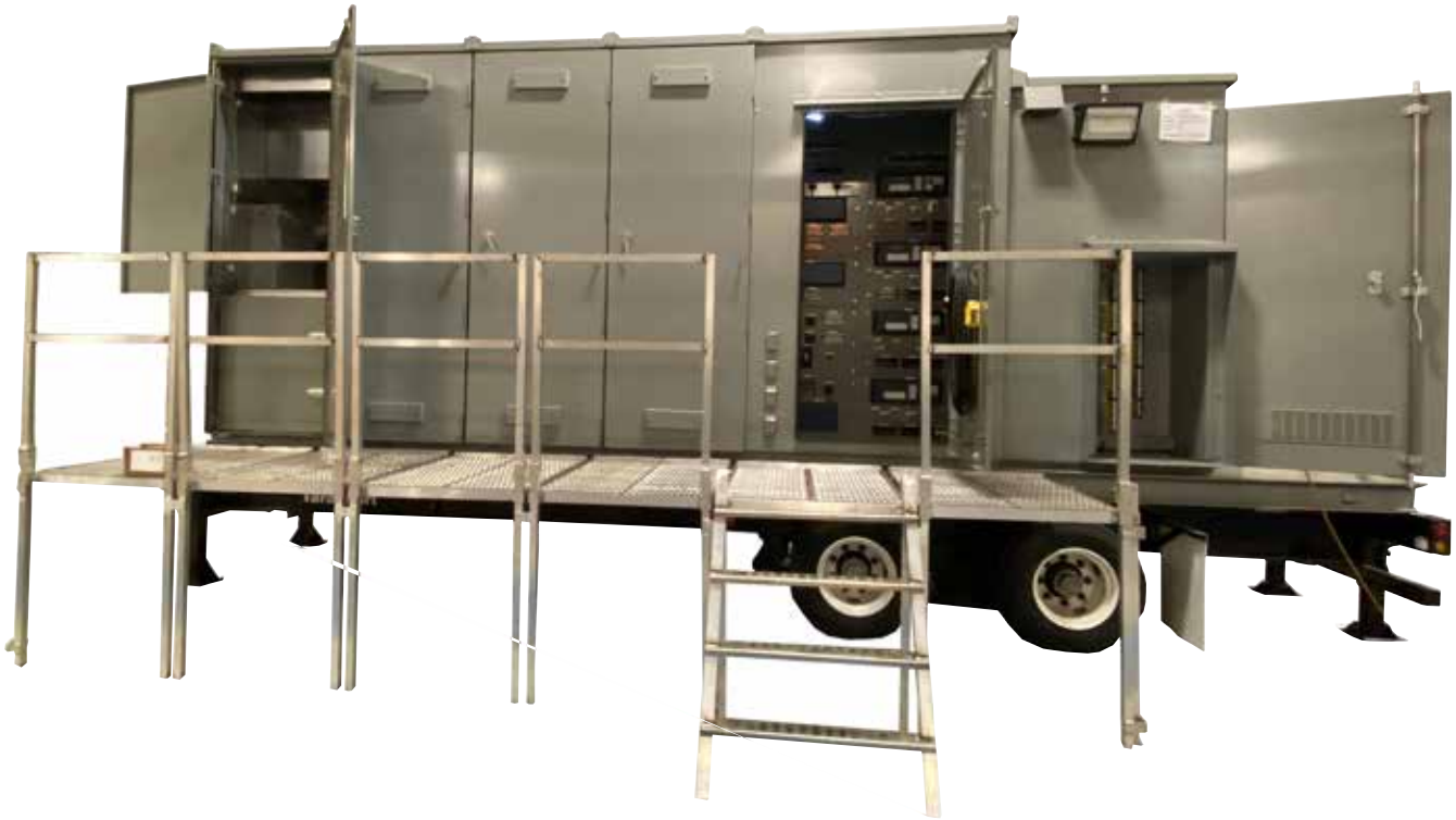
Operation side of the switchgear trailer. All circuit breakers and relays face this direction.
