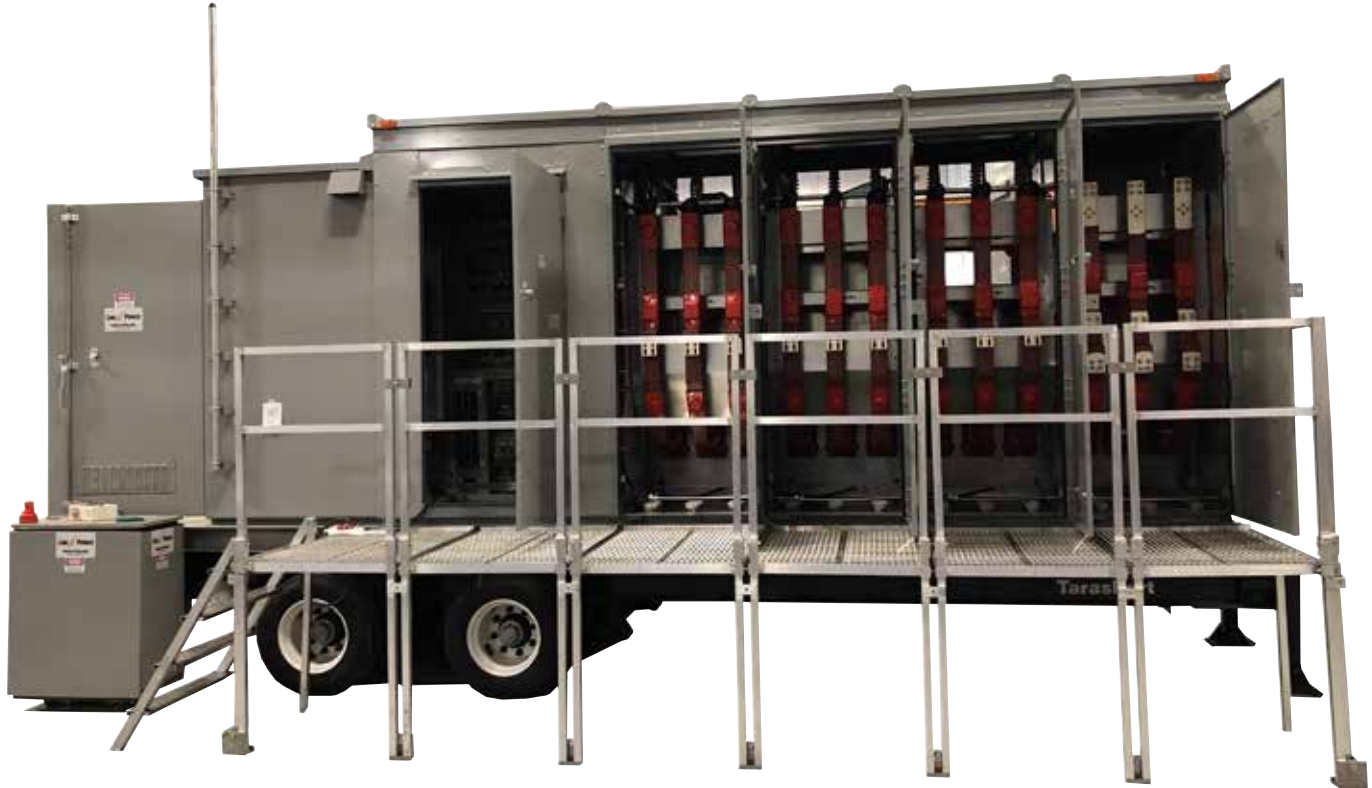
Rear View, revealing termination locations of MV cables, and access to the back of relays and low-voltage panelboards.
