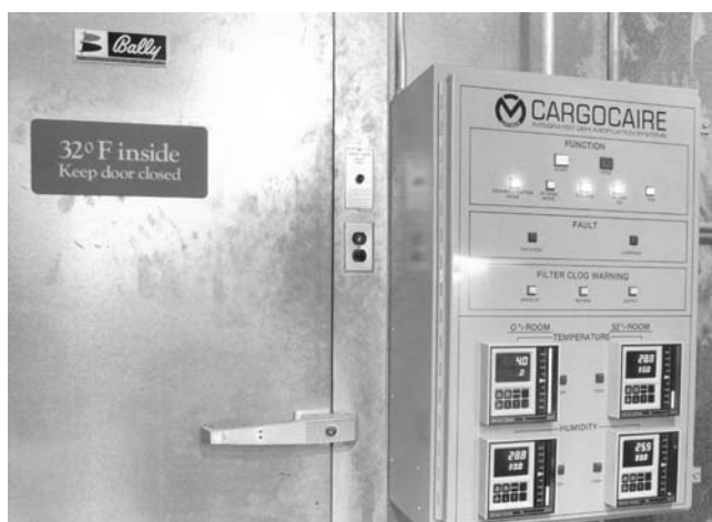
The 0°F vault for nitrate film storage is located inside the larger 32°F vault. The control panel on the right monitors temperature and humidity levels in both vaults.
