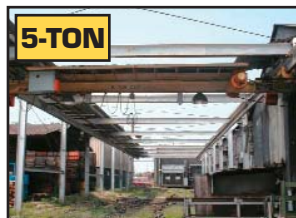
5-Ton MPH Bridge Crane
