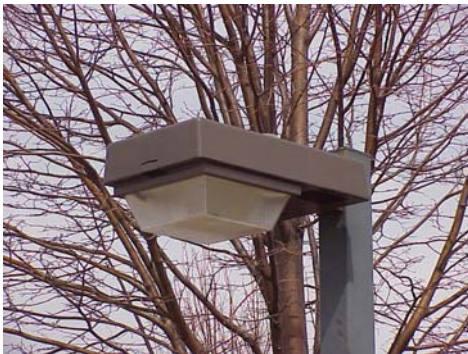
Rest Area Luminaires (Shoebox with Drop Lens)
