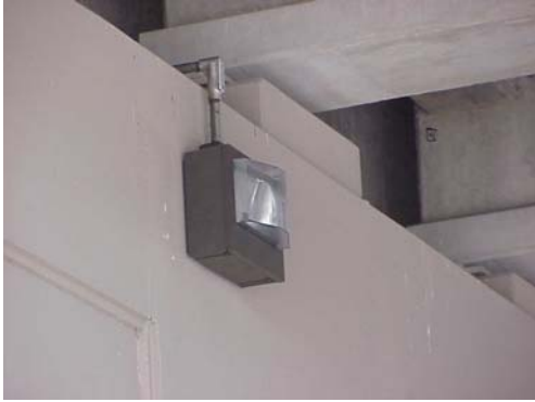
Bridge Underpass Luminaire
