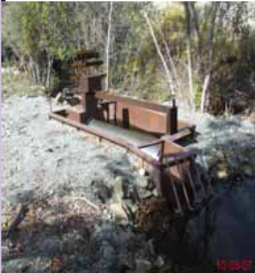
Modular screens such as the one above were installed on Howard and Targhee Creeks to prevent entrainment of cutthroat trout
