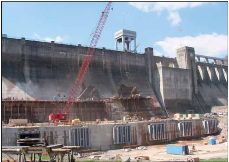
Work on the Bluestone Dam to bring the structure up to modern day safety standards has been ongoing for several years. Photo courtesy of CTL Engineering, Inc., South Charleston, who performed materials testing and construction services in conjunction with the U.S. Army Corps of Engineers.
