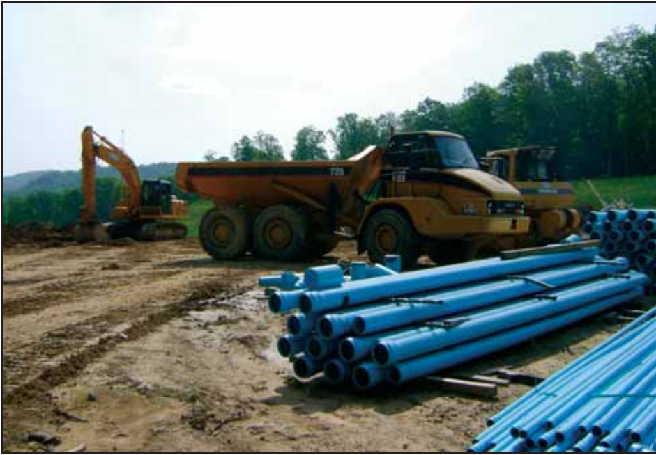
American Recovery and Reinvestment Act money was a big part of utility agencies funding in 2009 and 2010. With that money exhausted, water and sewer construction is expected to decline in 2012. Utility construction companies, such as Cook's Excavating, Pineville, pictured, are preparing for a decrease in projects. Water and sewer construction is essential to economic development and quality of life. Increases in funding are being discussed at the federal and state level.
