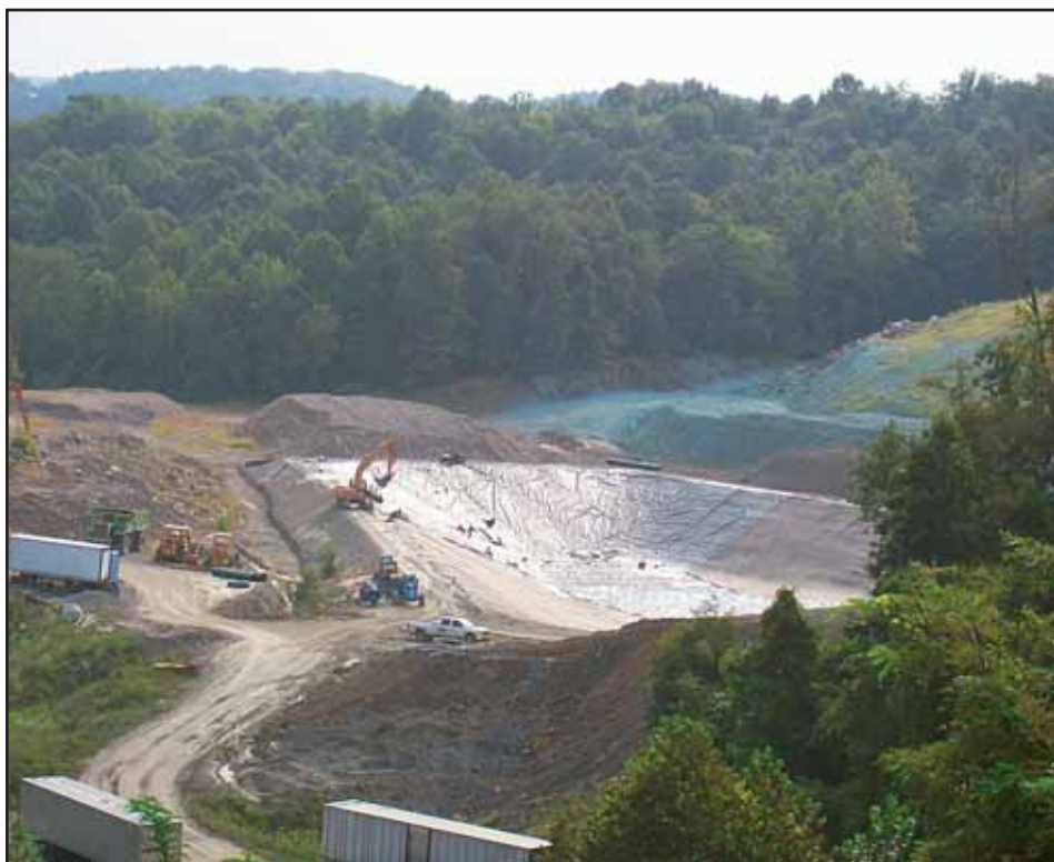
Oil and natural gas related projects, such as this impoundment pond, are expected to be a bright spot for construction in West Virginia in 2012, according to AGC of America. Bear Contracting, LLC, Bridgeport, completed this impoundment pond in Harrison County for PDC Energy.
