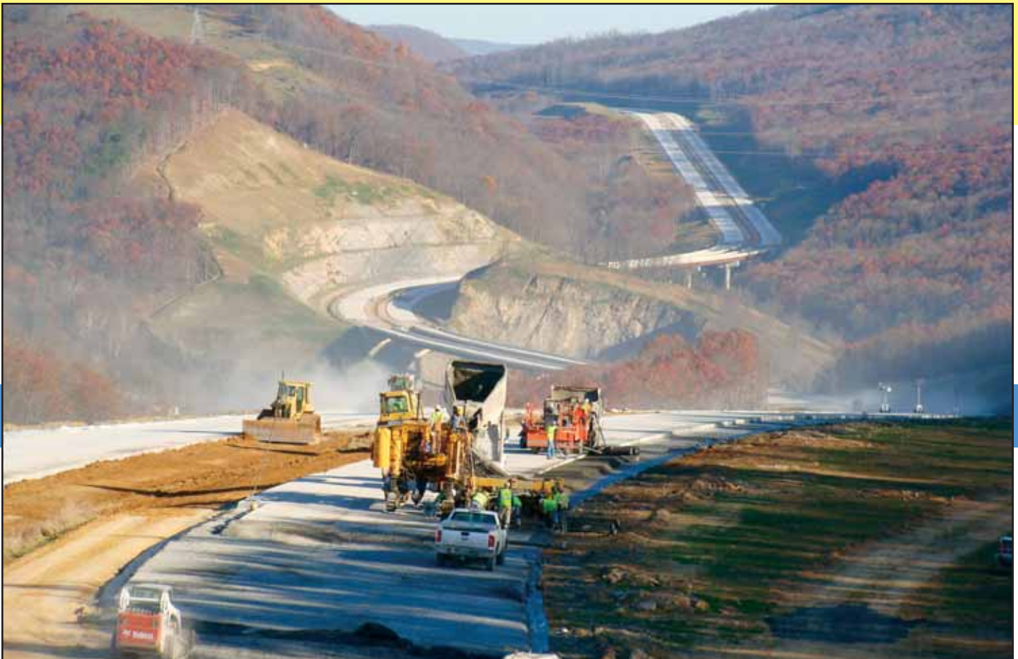
Hi-Way Paving, Inc., Hillard, Ohio, places concrete shoulders and shapes the median ditch along Corridor H in Grant County, near Scherr. The project bid in June 2011 and will be complete in 2013. When completed, Corridor H will stretch 130 miles from I-79 at Weston, cross the border into Virginia and travel 13 miles to meet the junction of I-66 and I-81. The 130 mile stretch within West Virginia is 75 percent complete or under construction and by 2018 that number should increase to 87percent. Photo courtesy of Mike Durst, Hi-Way Paving, Inc.
