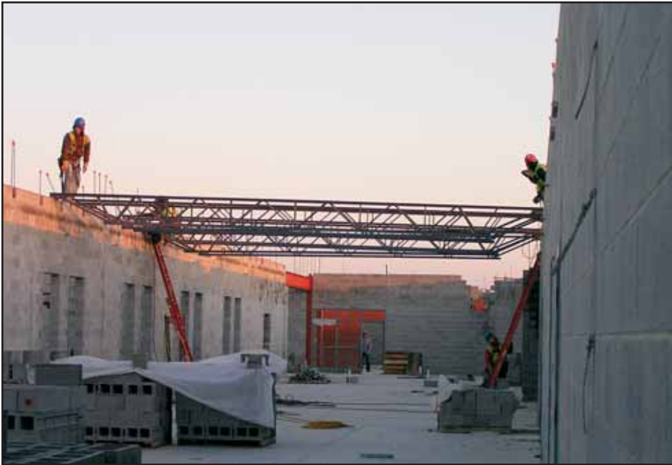
Workers install second floor joists in the academic wing at Spring Mills High School in Martinsburg. Photo by Bill Ratcliffe, Williamson Shriver Architects.
