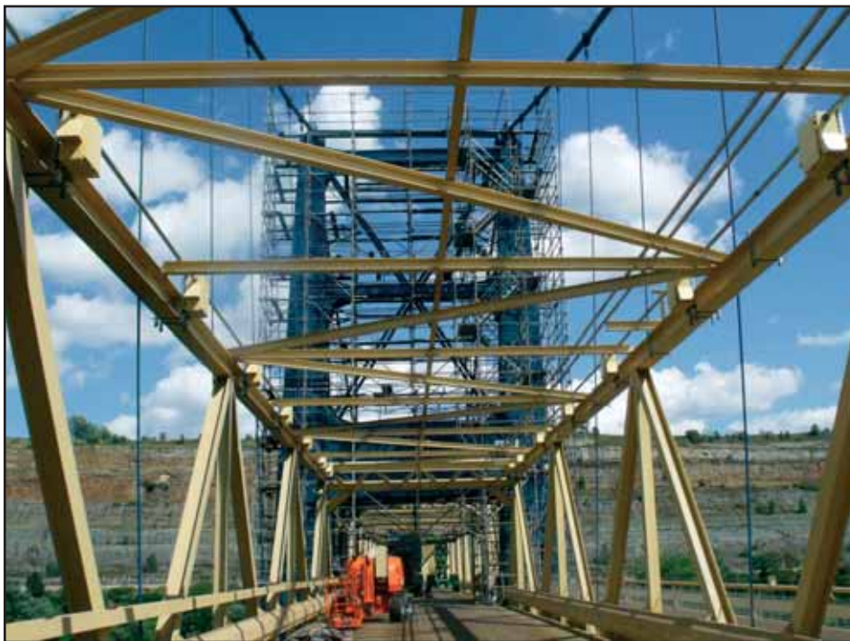
The Market Street Bridge, which connects Follensbee, WV, with Stubenville, OH, was opened in December 2011 following nearly two years of rehabilitation work. Ahern, a Division of Kokosing Construction, South Charleston, was awarded the $16,547,000 contract in November 2009, which included repairs to the structure, cleaning, painting and aesthetic lighting.
