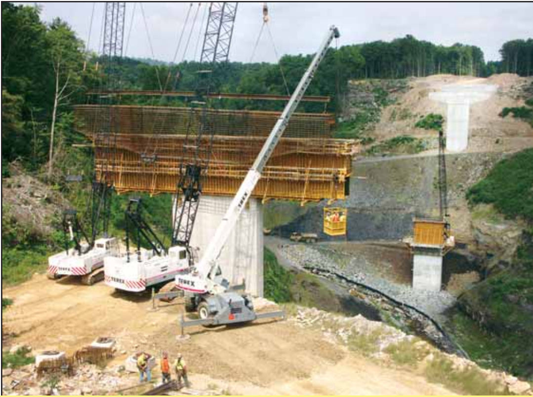
Crews with Vecellio & Grogan, Inc., Beckley, overcame challenging conditions to build the final two segments of a Route 19 bypass highway just east of Beckley. Vecellio & Grogan constructed a 1,200-foot bridge over a steep, 217-foot-deep gorge with limited access for equipment. Crews also built 1.6 miles of four-lane highway leading up to the bridge and rejoining with local traffic on the other side. Photo by Carl Thiemann, Communications Director, Vecellio Group, Inc.
