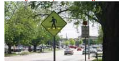
Rectangular Rapid Flashing Beacon
