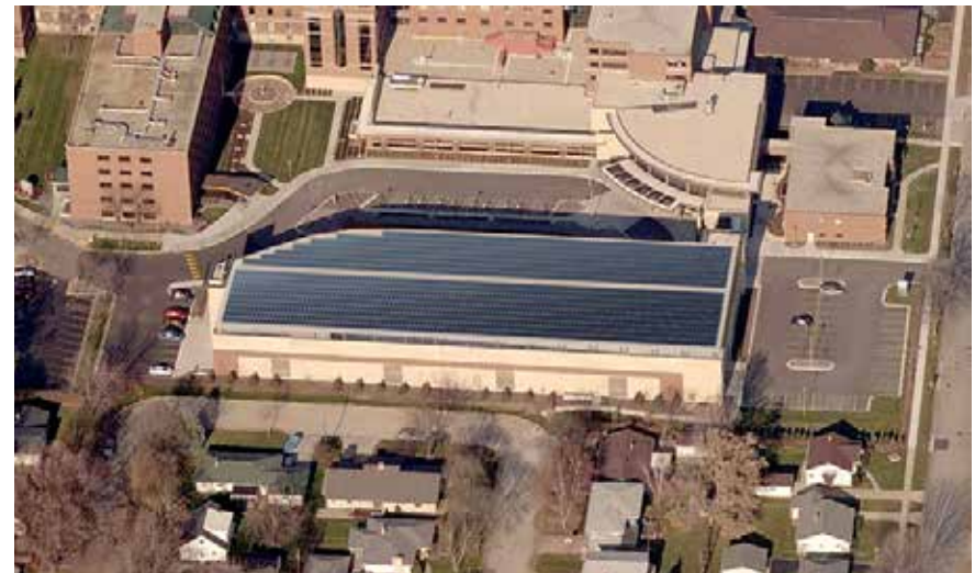
Figure 5-4 Photovoltaic Installation on Parking Garage, St. Elizabeth Hospital, Affinity Health, Appleton, WI
