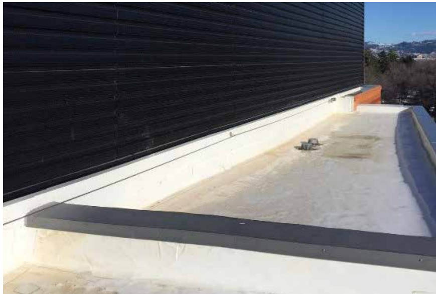
Figure 5-2 Transpired Solar Collector Installation, Montana State University Jake Jabs College of Business & Entrepreneurship
