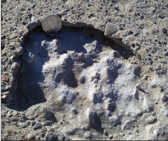
Pit in concrete
