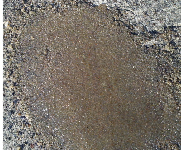
Pit patched with epoxy and sand
