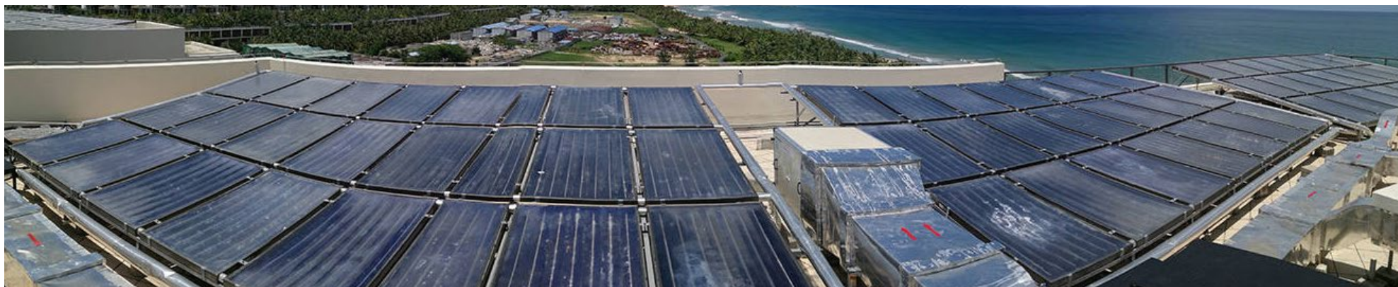
A solar panel installation in action at the Xiangshui Bay Marriott Resort & Spa, Sanya, China.
