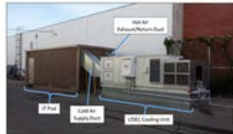
UTA's research modular data center facility in Dallas, Texas
