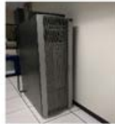
Cisco Liquid Cooled Servers
