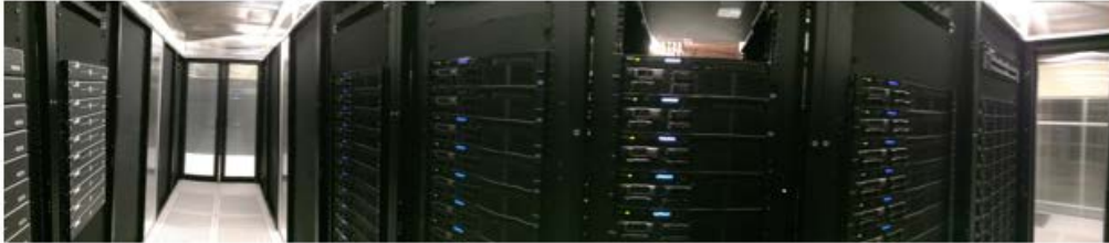
Panoramic view of one of the cold aisles in ES2 Data Center Laboratory at Binghamton University
