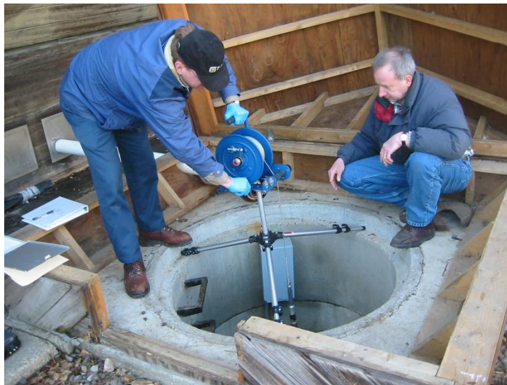
IBM employees use a televIEWing system to assess performance of a groundwater extraction well.
