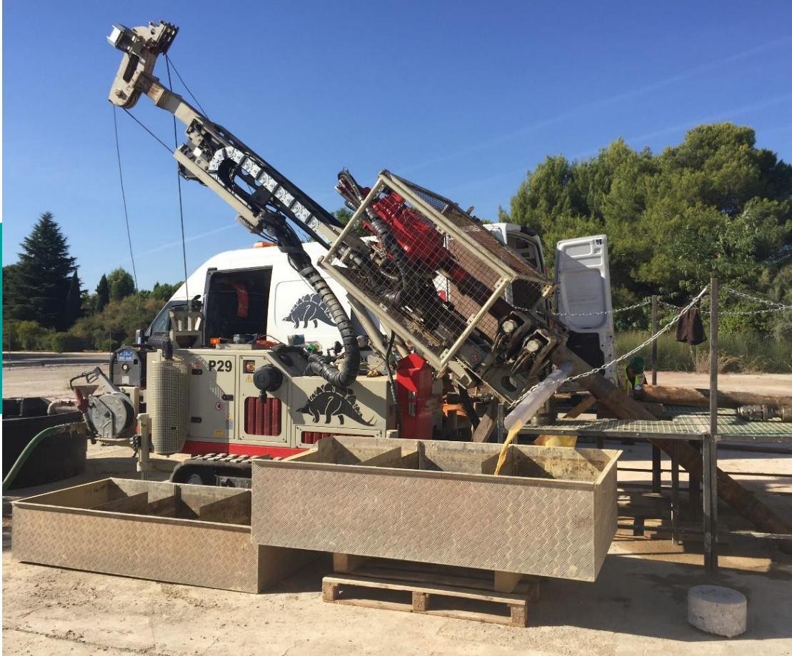
Installation of a groundwater monitoring well at the former IBM Montpellier, France, site.
