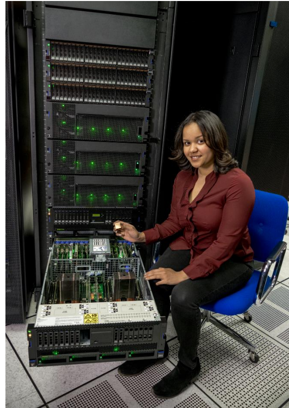
IBM engineer Ana Santos De Leon tests an IBM Power Systems server in Austin, Texas.
