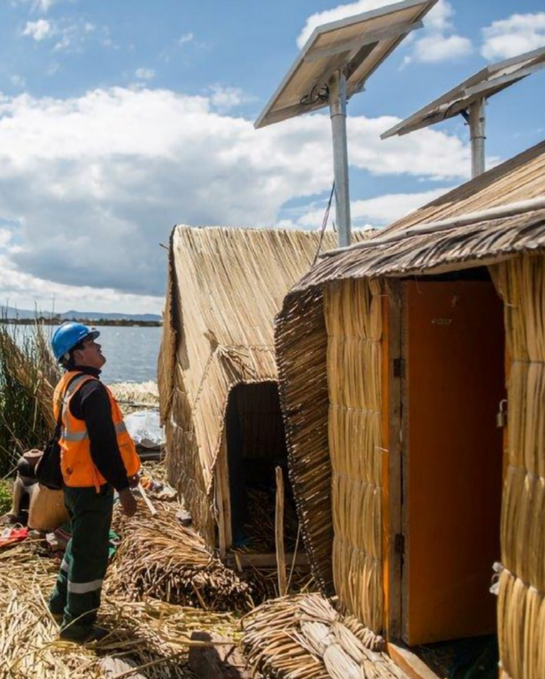
Off-grid solar renewable energy project, Peru. Photo provided by Ergon.
