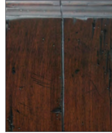
MEDIUM DISTRESS Shown on Plank Top
