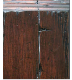
HEAVY DISTRESS Shown on Plank Top
