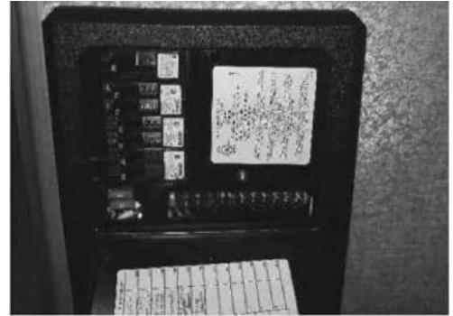
Figure 9-9 Main 120 VAC Load Center
