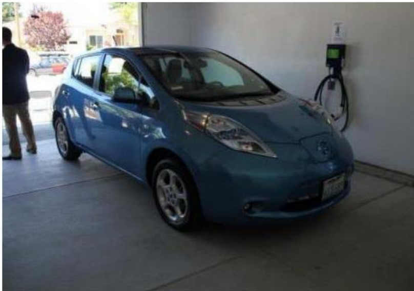
Figure OR-7. Electrical Outlet Ready for Electrical Vehicle Service Source: basc.pnnl.gov/images
