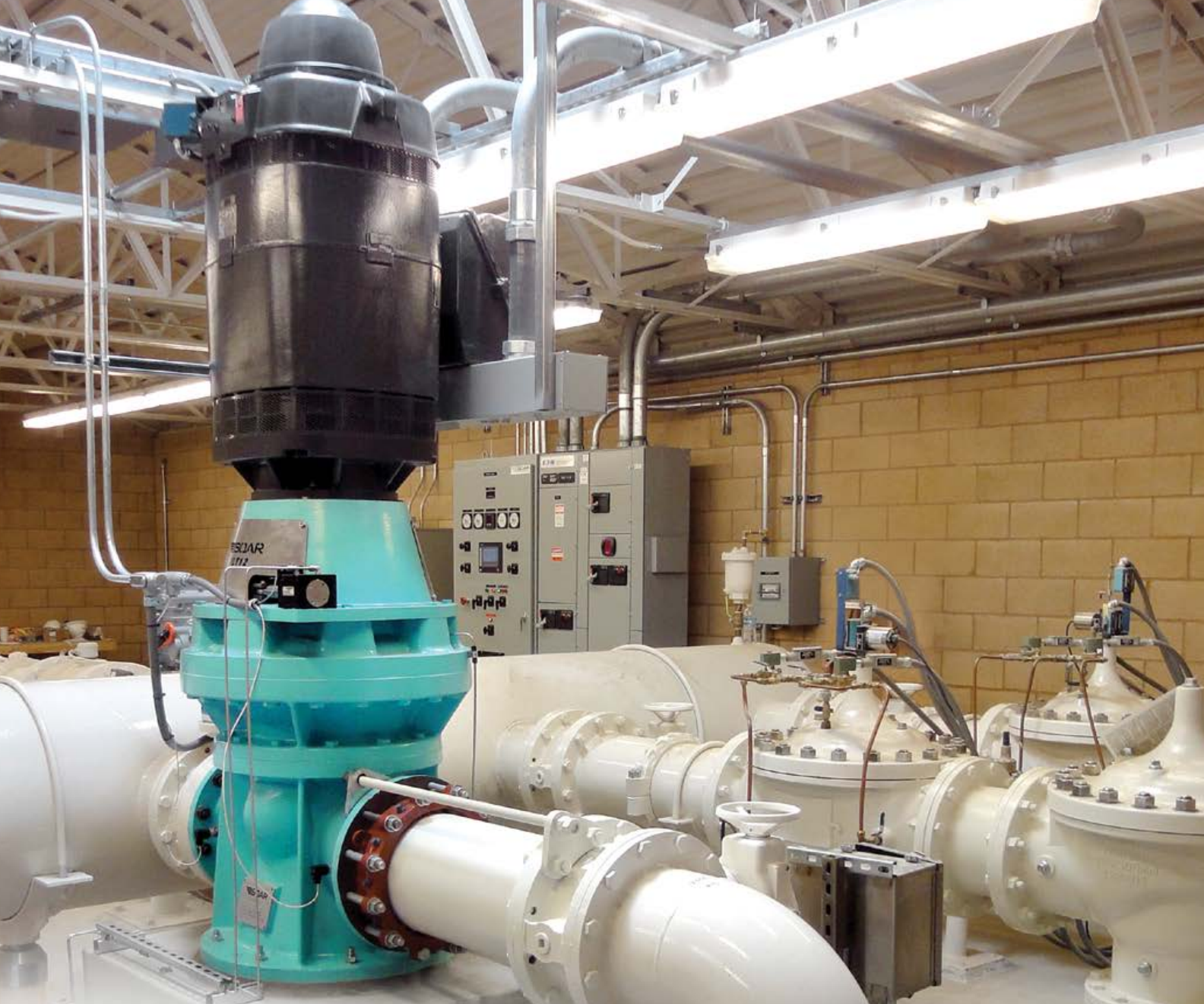
208 kW Variable Flow In-Line Turbine
