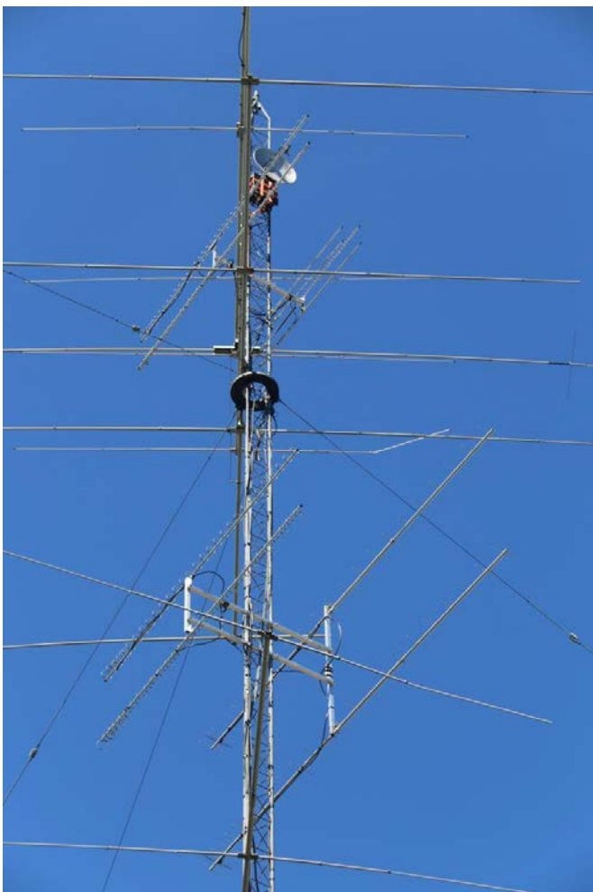
The N2WK UHF/SHF Rotating tower array – all bands from 432 MHz – 10 GHz – nice! (Photo Courtesy: Ronald Craig, N5BNO, from QRZ.com )
