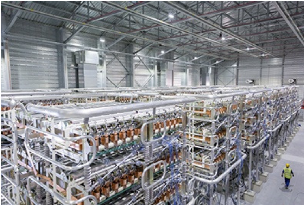
Figure 3: HVDC Converter Hall for 320 kV 2 GW VSC Transmission Link
