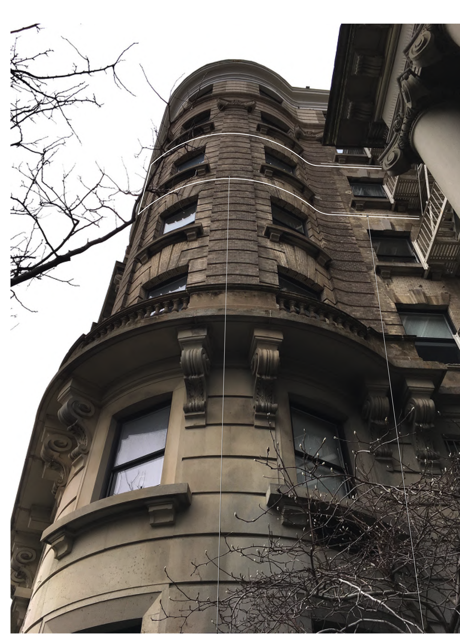
WINDOWS TO BE REPLACED, APT. 508/509
