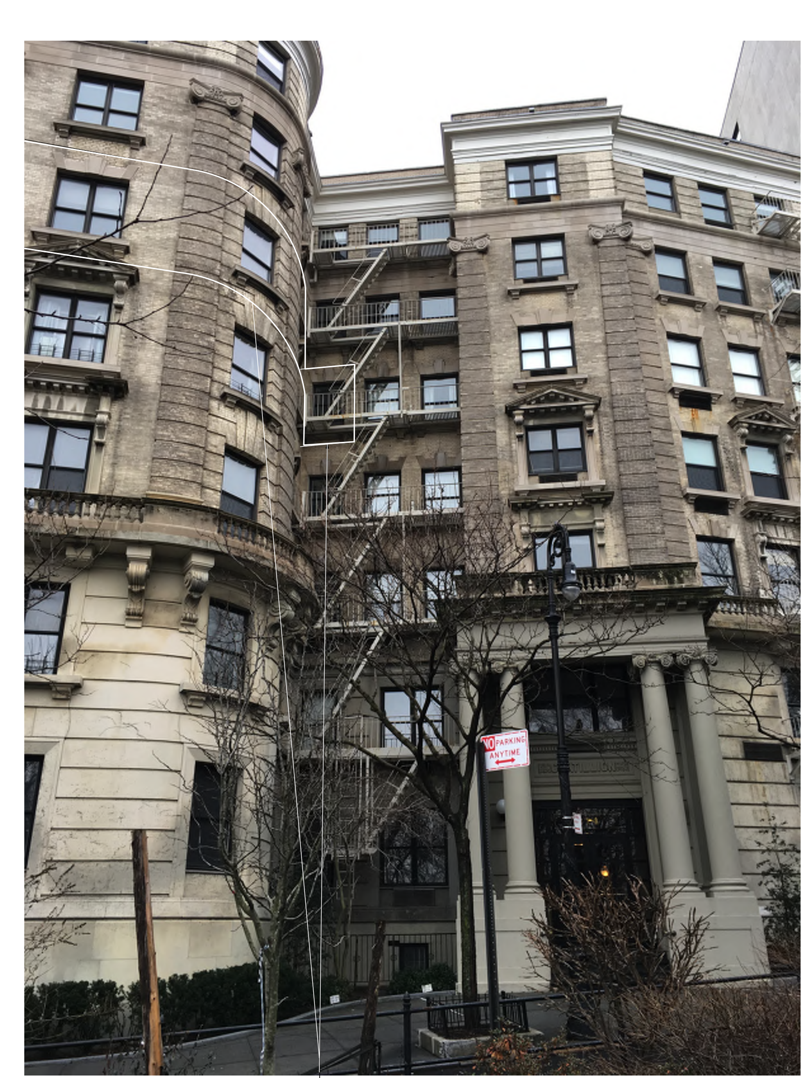
WINDOWS TO BE REPLACED, APT. 508/509
