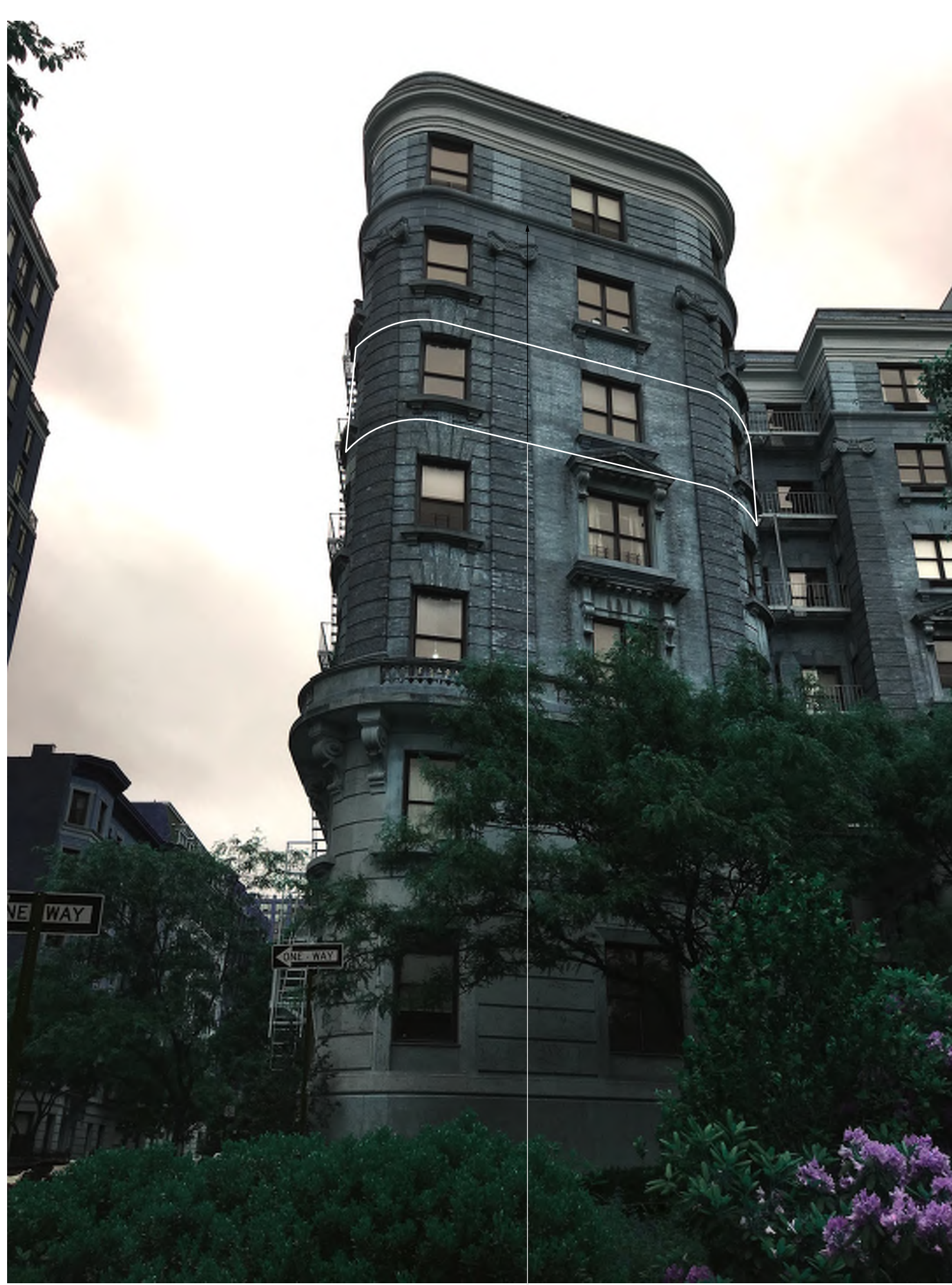
WINDOWS TO BE REPLACED, APT. 508/509
