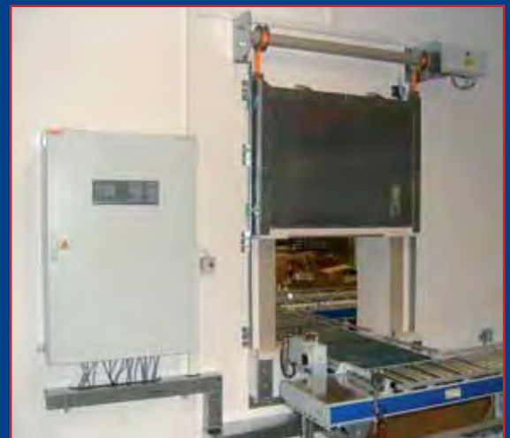
Continuous belt conveyor with 480 VAC emergency power system
