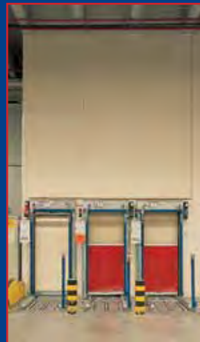
Conveyor system forms ceiling-high wall
