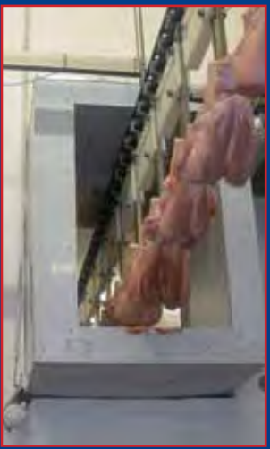
Overhead conveyor for e.g. chicken
