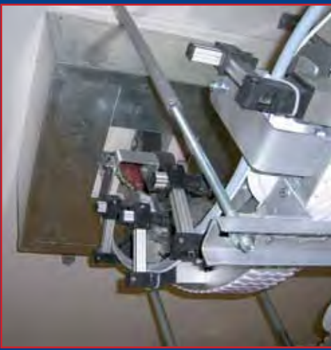
Hinge chain conveyor through ceiling openings
