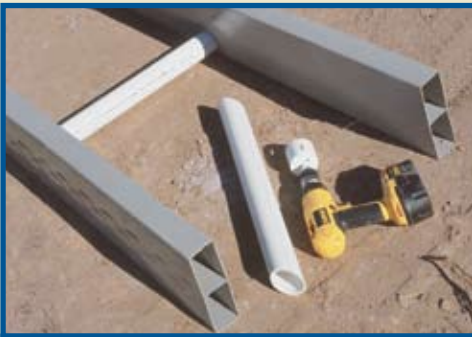
PVC PIPE/DRILLED HOLES
