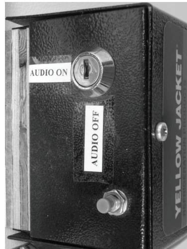
On/Off positions for key to turn off sounder when in alarm.
