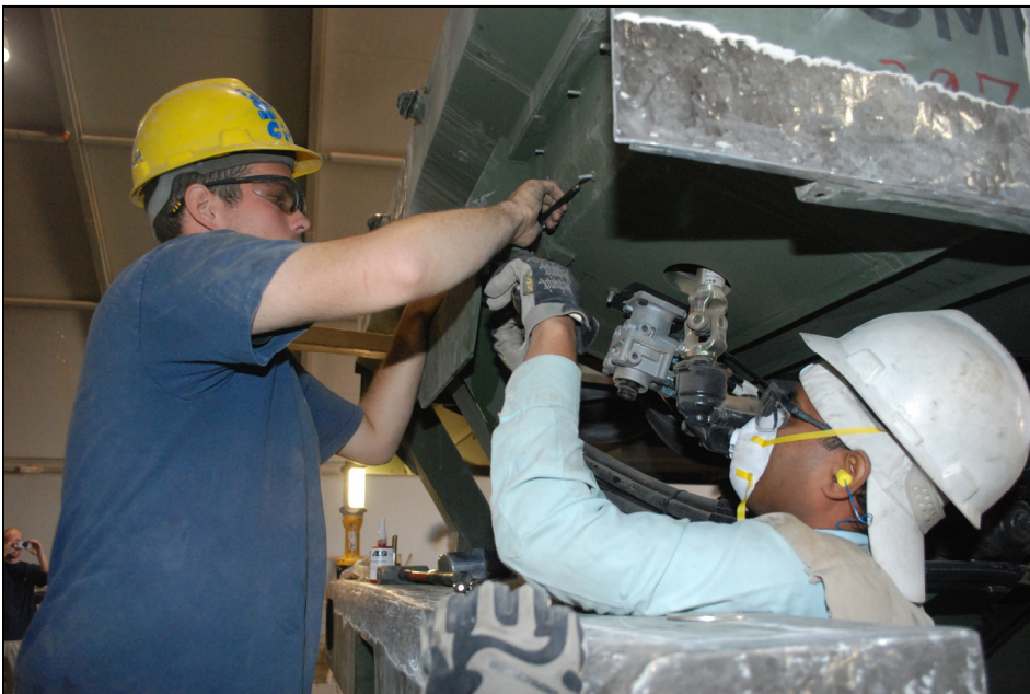
Michael Woodall, a contractor with URS Corporation (left) and Prahlad, who uses one name, a subcontract worker with Kulak Construction Company, install cab mounts on a TEREX MAC-50 Crane.
