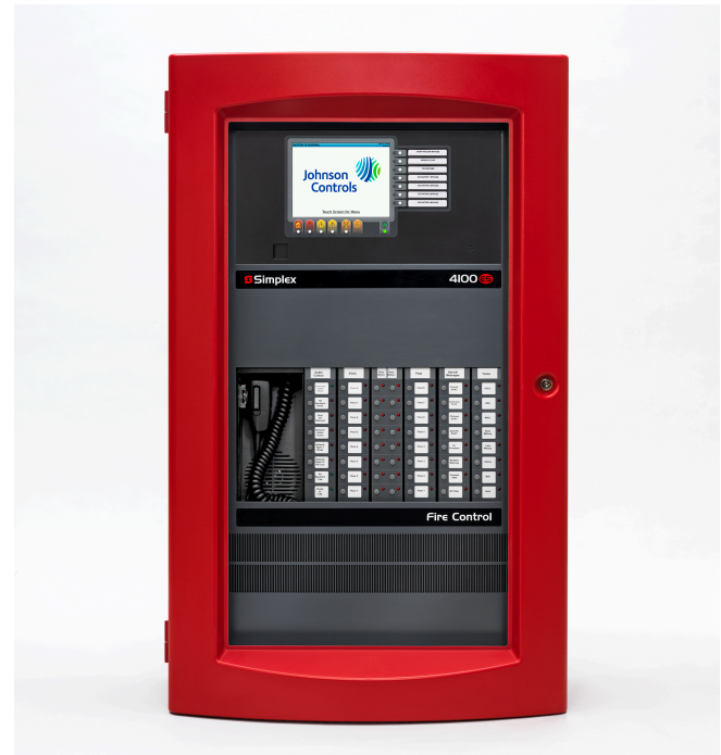
Figure 1: 4100ES Fire Alarm Control Panel with ES Touch Screen Display and Voice Options
