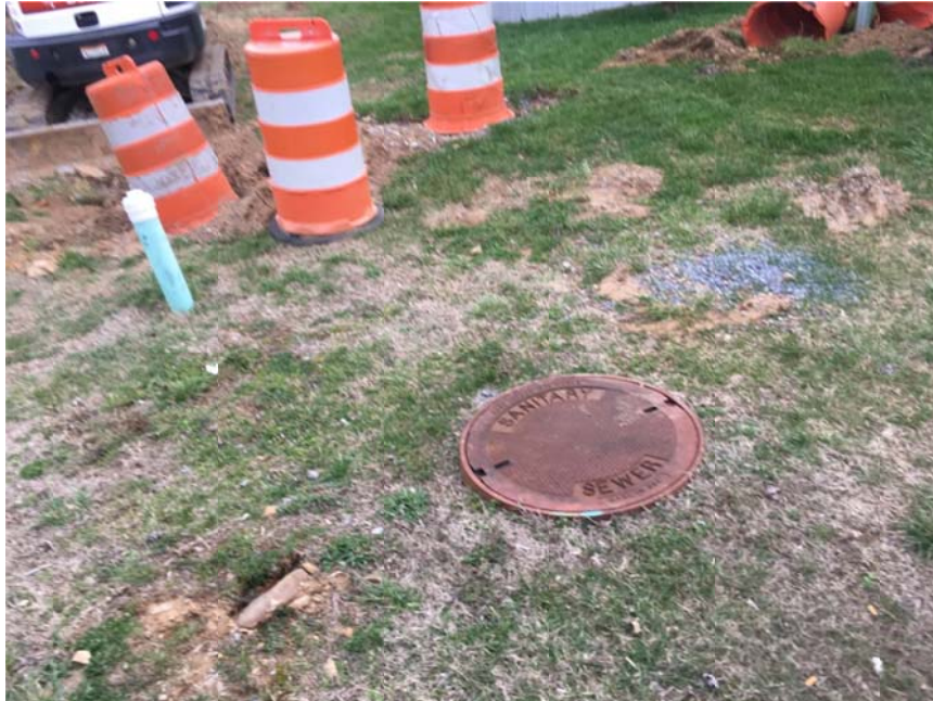
Sewer lines connected to city sewer system.
