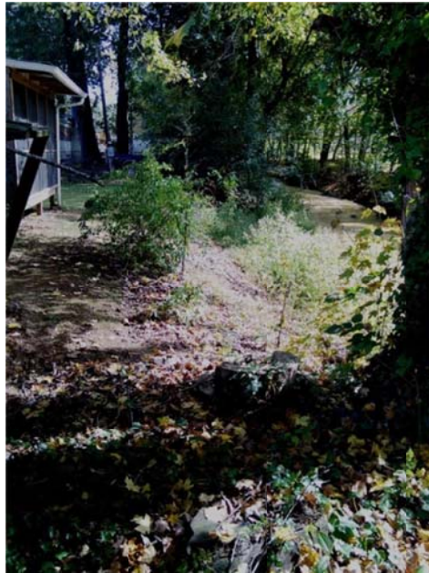
Mobile home next to Gap Branch (After stream stabilization in previous project and before current project of septic system removal & sewer connections).
