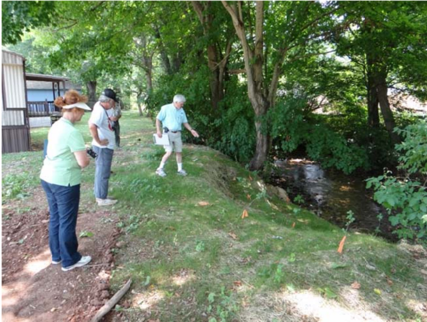
This site of 25' in length was a 3' high, eroded, bank. It required sloping along with matting, grass and tree plantings.
