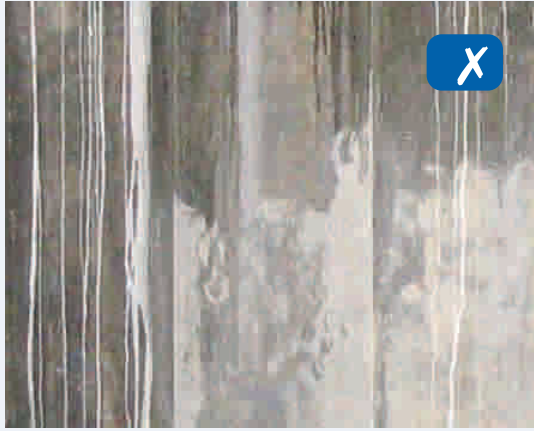
Presence of form oils with efflorescence
