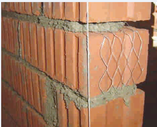
Mesh reinforcement embedded at every 4 th course and tucked into the next course
