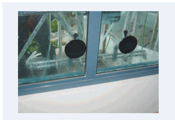
Figure 6.1: Conduct of field watertightness test for joints between external wall and window frame
