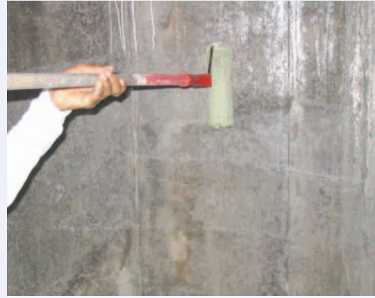
Application of cleaning solution to remove residual form release agents on concrete surfaces
