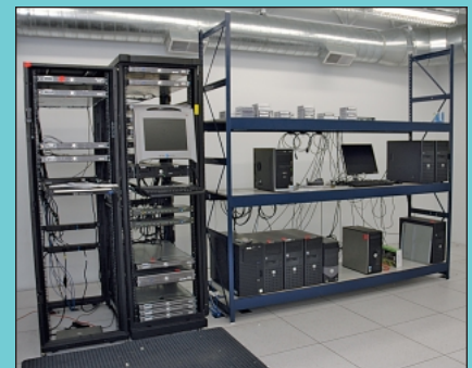
Overall View Server Room Including Server System and Infrastructure w/ Raised Floor Air Handler & Fire Suppression System
