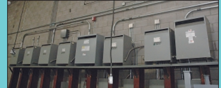
**Overall View (9) Late Model Transformers
