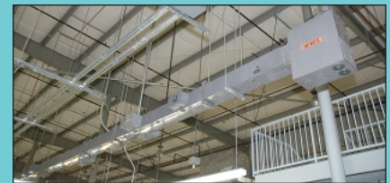
**160' Square D Catalog No. APD-3080-515 Copper Plug-In Bussway
