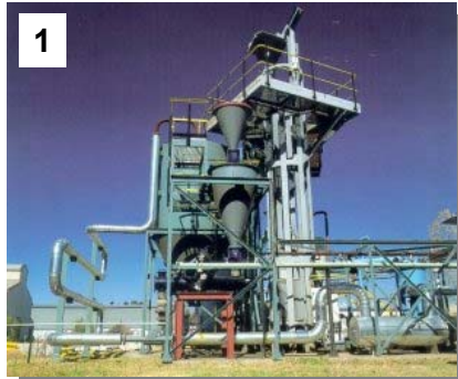
1 Pneumatic conveyor / drier
