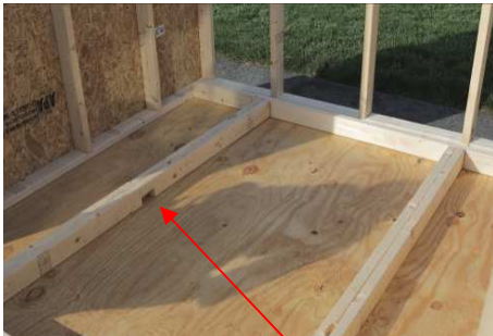
(49) Place the door studs as shown, making sure to have the notch for the door latch facing down, and on the left door jack as shown.
