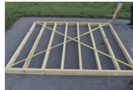
(17) Before proceeding with flooring, ensure that floor is square. Both measurements need to be equal.
