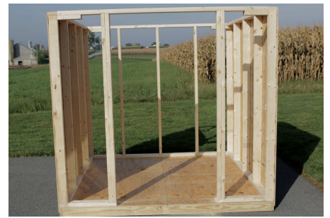
(51) Set the front gable wall, and fasten to floor and side walls as done in previous steps, and making sure to space the bottom of the door opening the same as the top, which should be 39-1/4”
