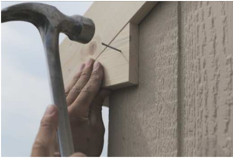
(100) Fasten a bird box block to the corner, using three 2” Trim nails.
