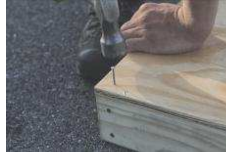
(23) Now; nail front left corner, again; making sure flooring is flush with the band board.
