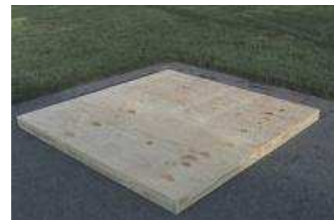
(26) Finally, make sure flooring is nailed to all floor joists, then you are ready for wall placement.
