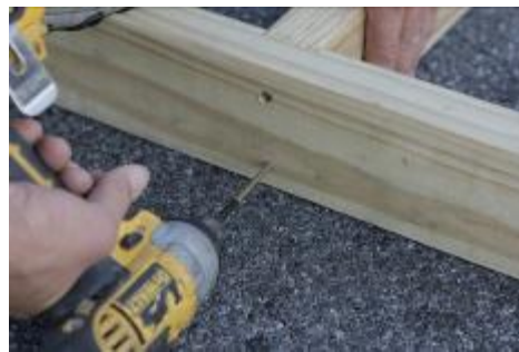
(16) Continue this method for rest of floor joists, using two 3" screws per joist. *Holes are predrilled*
