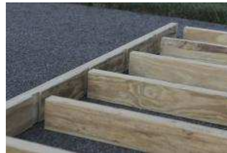
(14) Note: The band boards have dado grooves precut to ensure proper joist placement.
