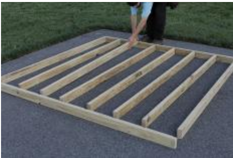
(13) After making sure the pad is level, locate the parts to assemble the floor joists, and scatter them out as shown.
