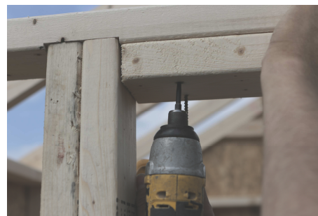
(53) After walls are all fastened, locate the 39-1/4” long 2x4, place it under the door top plate as shown here, and fasten with six 3” screws.
