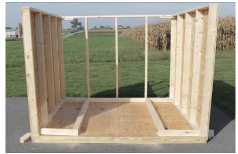
(48) Now; locate and lay out the parts to assemble the front wall.
