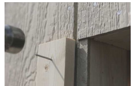
(108) Now; install left side door trim, staying flush with the top of the door frame. NOTE: Trim spacing needs to be 40-1/2” (inside to inside) as shown in next step.
