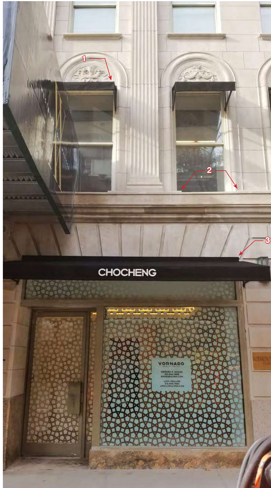
DETAIL MOCK-UP PHOTO: TAKEN FROM EDGE OF SIDEWALK ON MADISON AVE. LOOKING UP
