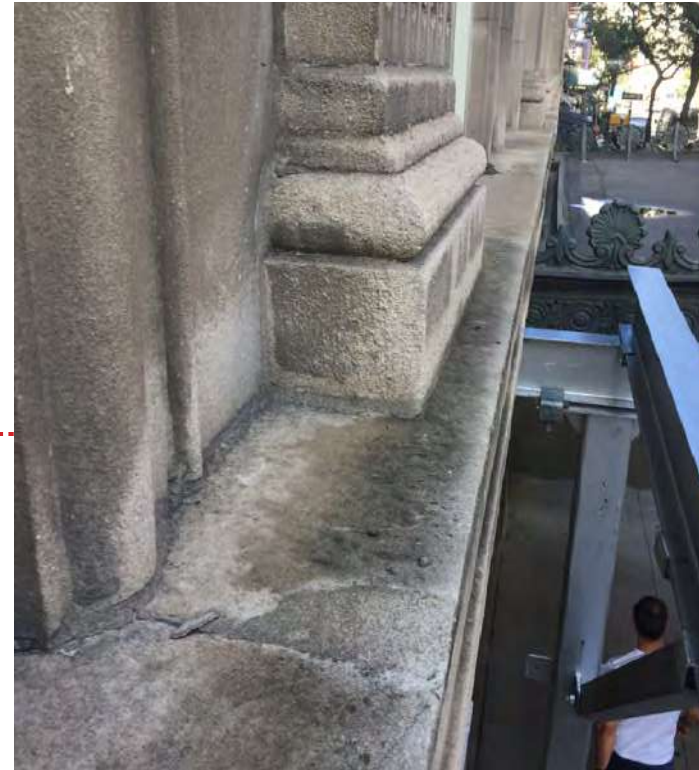
PHOTOS FROM OUT THE SECOND FLOOR WINDOW TO THE LEDGE (FLUTED PIER)
