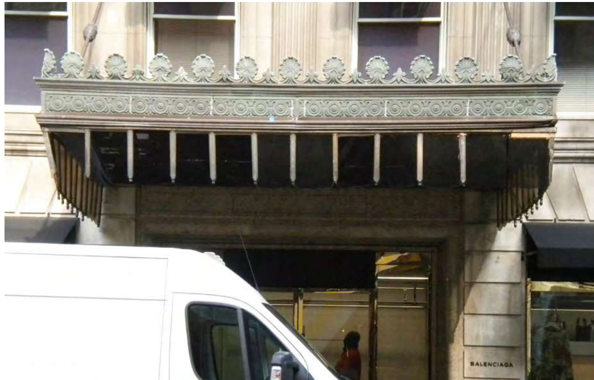
EXISTING MARQUEE ON MADISON AVENUE (ELEVATION) (FRONT SECTION OF ACRYLIC SKIRT AND SUPPORTING ELEMENTS ARE SEVERELY DAMAGED OR MISSING)
