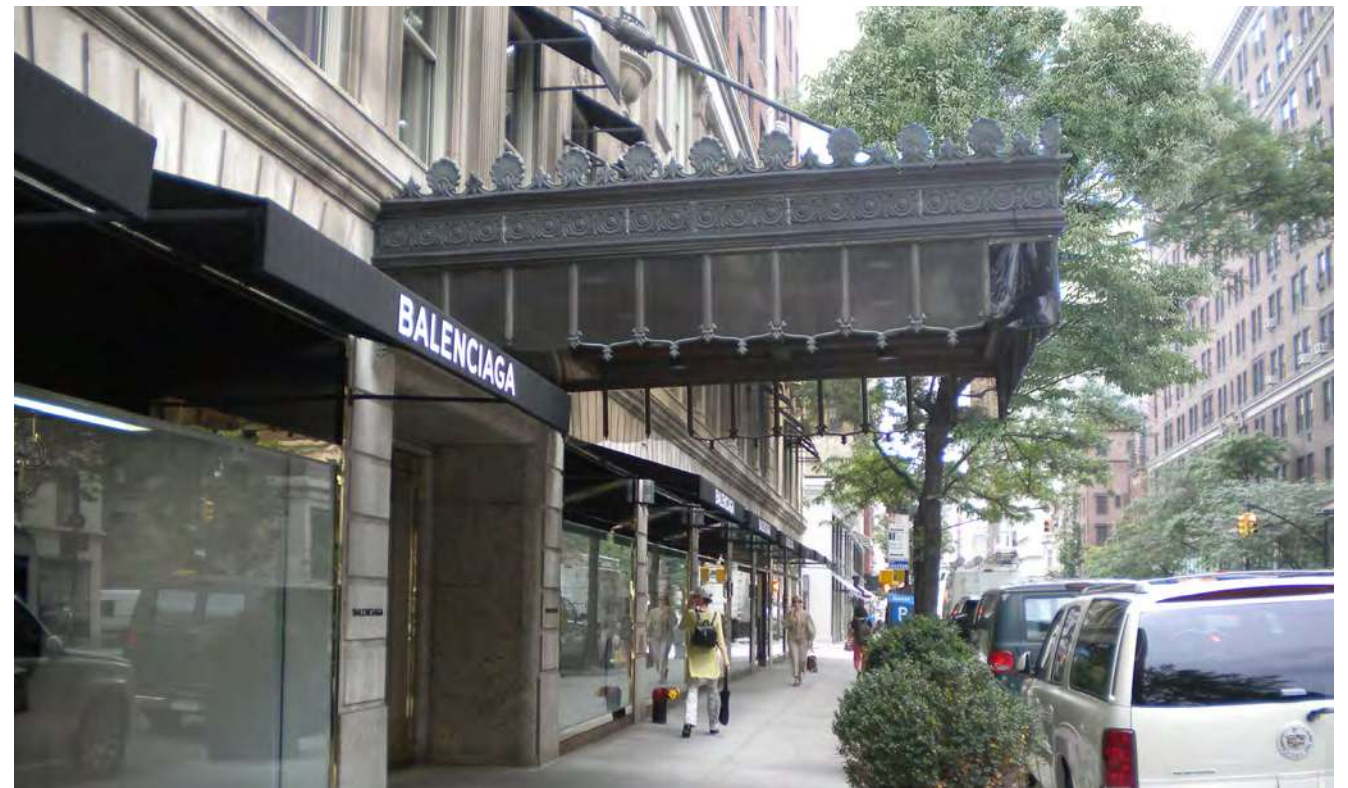
PERSPECTIVE VIEW FROM MADISON AVENUE - EXISTING MARQUEE (MARQUEE IS SEVERLY DETERIORATED & DAMAGED)
