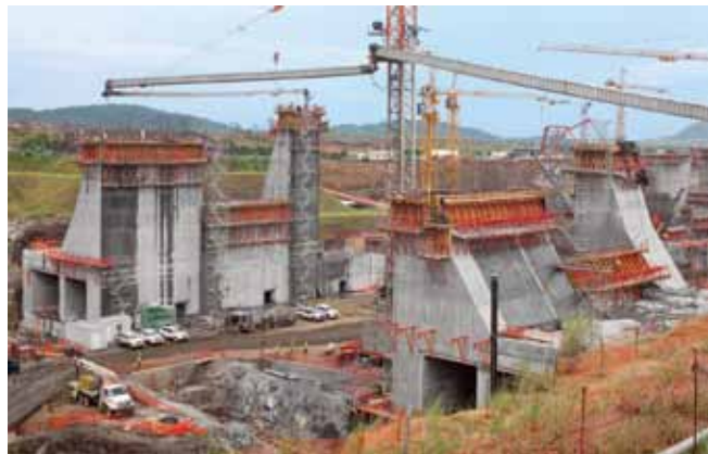
PERI is supporting the "construction project of the century" with the planning and delivery of huge quantities of formwork and scaffolding systems. Photo: PERI GmbH
