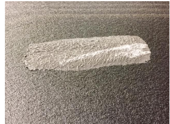
Sealant *Raised material, not a flaw
