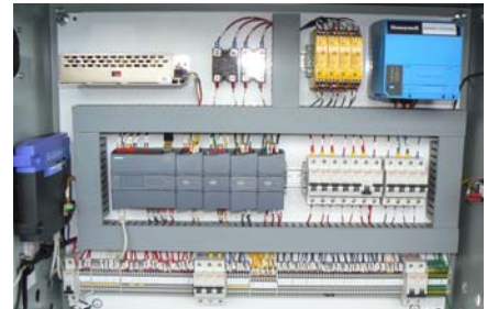
Standard Control Panel with Siemens S7-1200 PLC, Safety Controller, automatic circuit breakers, Ethernet Router, and Honeywell Flame Safeguard.
