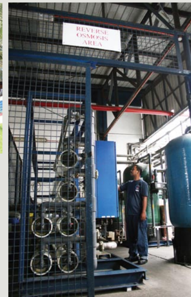
Reverse osmosis plant in Lipa Factory
