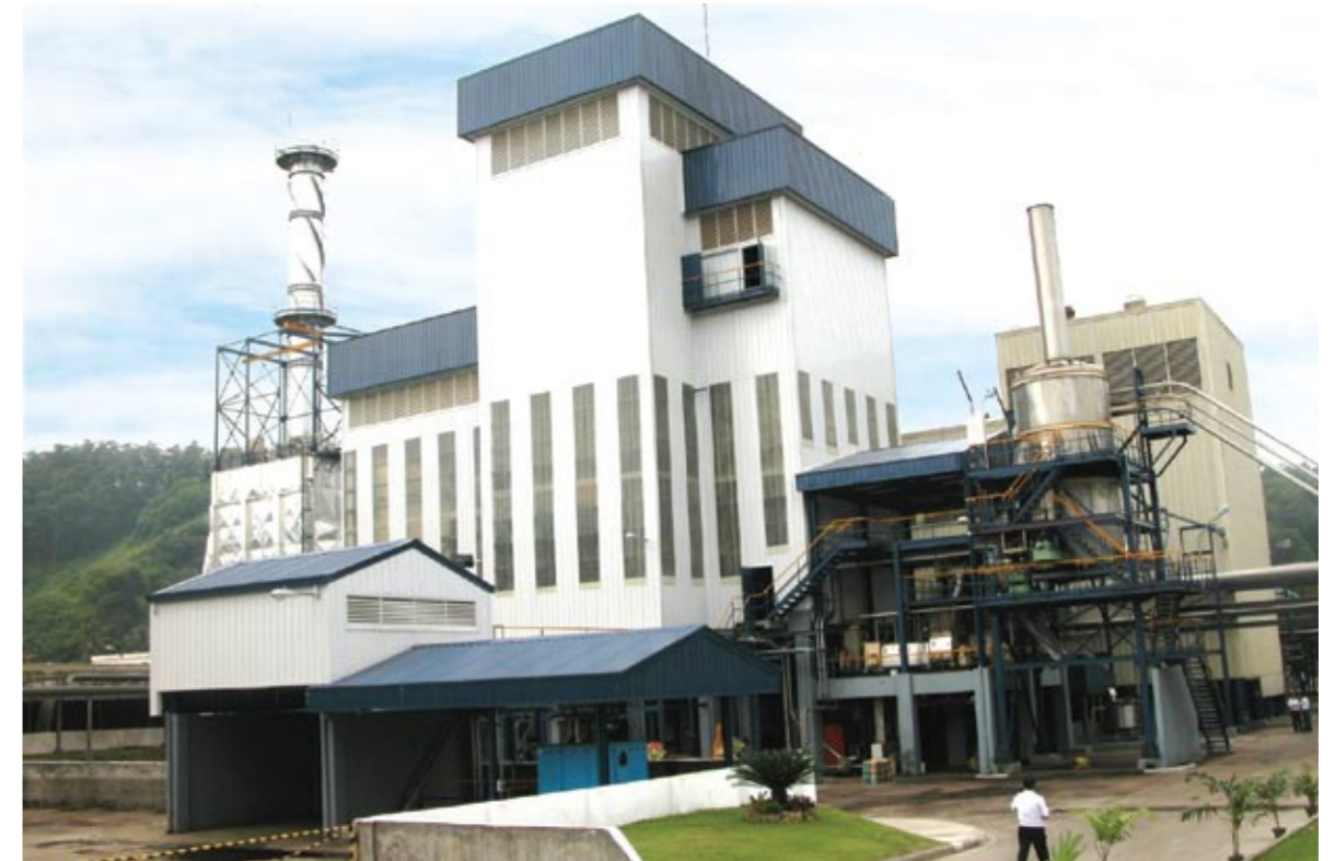
The Atmospheric Fluidized Bed Boiler in CDO Factory, which converts spent coffee grounds into steam
