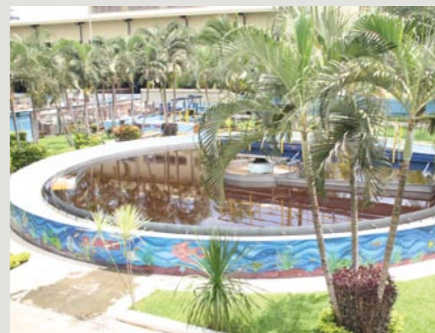
Exterior of the CDO wastewater treatment pool is painted with designs created by employees' children
