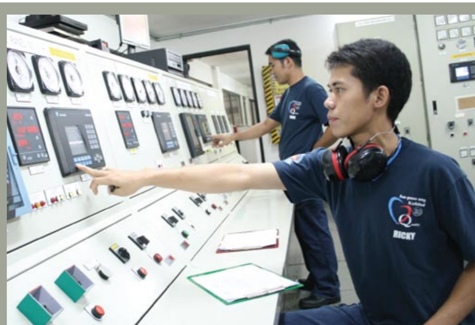
Key departments in the factories are installed with their own energy metering devices to closely monitor their consumption
