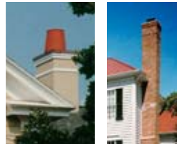
Acceptable stucco and brick chimneys with appropriate chimney cap.
