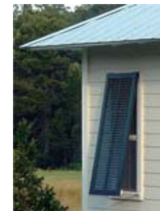
Operable Bermuda shutter in the open position.
