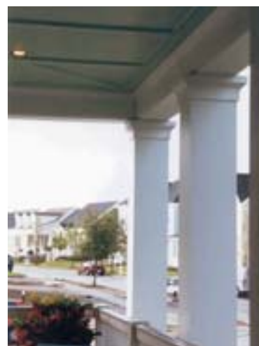
Free standing square columns with independent porch railing. Appropriate column to beam and soffit detailing.
