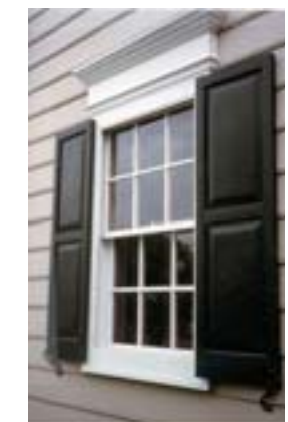
Acceptable operable shutter design in the pen position. Operable 'shutter dogs' hold the shutters in place.
