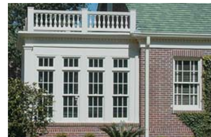
Double hung 6 over 6 windows with transoms and classical trim detailing and 6 over 6 double hung window with soldier course header and appropriate brick surround.
