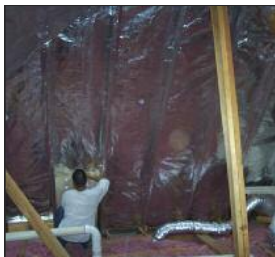
Aluminum foil deflects heat from attic. (courtesy)
