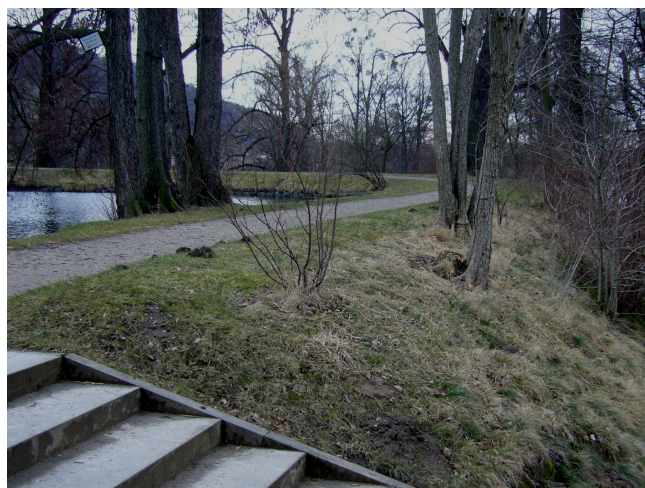
Figure 6: Shrubs rooting into the static Cross-Section of a small Dam (Photograph: Pohl)
