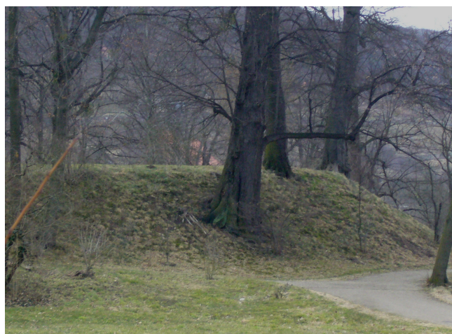
Figure 5: Trees rooting into the static Cross-Section of a small Dam (Photograph: Pohl)
