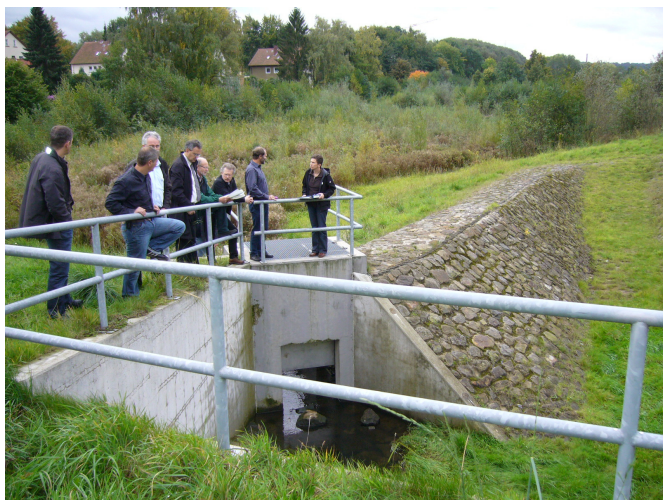
Figure 4: The Members of the technical working Group visiting the Spillway Section and Bottom Outlet of the small Dam of the Flood Control Reservoir Hainteichstraße/ Gellershagener Bach in Bielefeld (green reservoir, storage volume < 30,000 m 3 , Photograph: Pohl)
