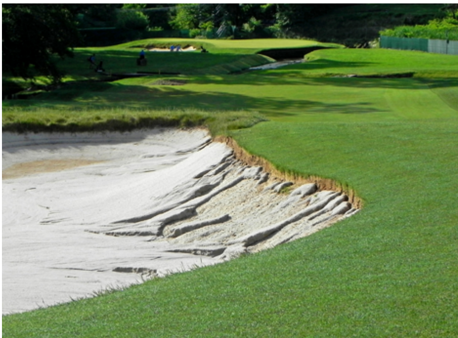
Reducing washouts is one of the primary reasons to install bunker liners. Washouts are time consuming to repair and can contaminate bunker sand.
