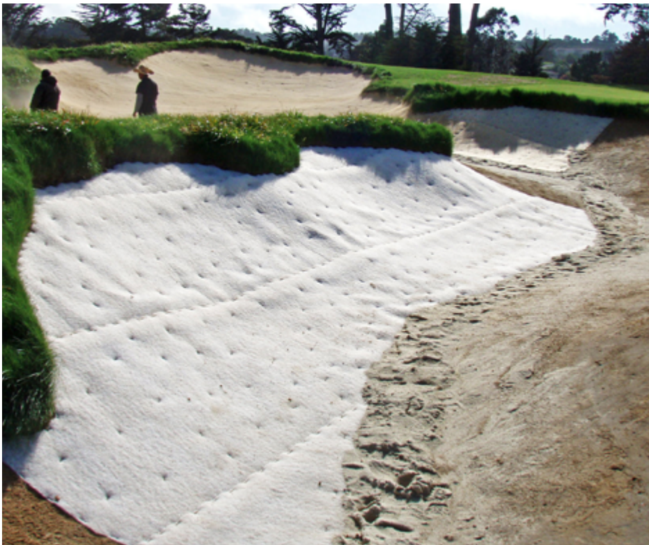
Fabric liners help prevent washouts on steep bunker faces, but they can be easily damaged by maintenance equipment or animals.
