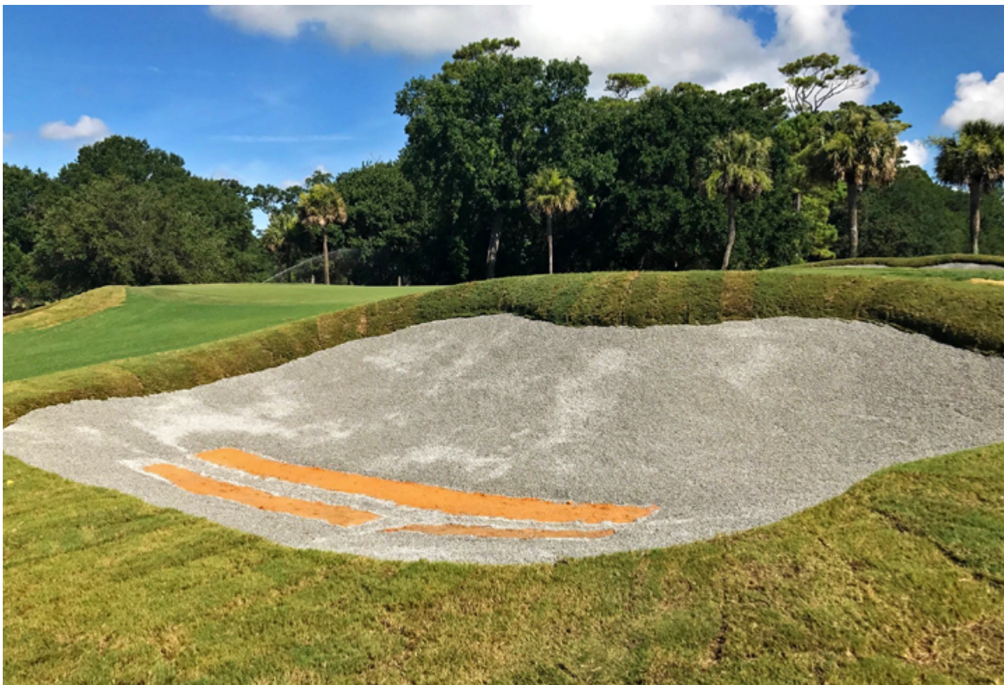
When using porous aggregate liners, some facilities have elected to leave gaps in the liner to prevent a perched water table from causing excessive sand moisture.
